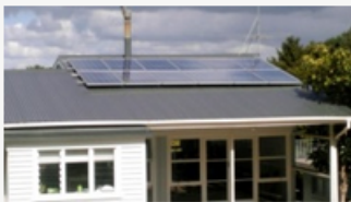
Solar power (PV)
