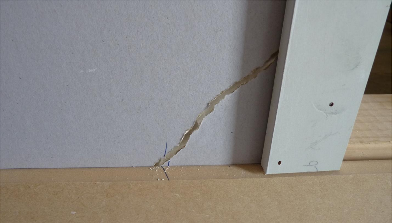
Photograph A.6. Plasterboard crack on the 3.6 m long wall on Side 2 formed after regime Long 3 (nominal 12 mm) taken after regime Long 5 (nominal 23 mm)
