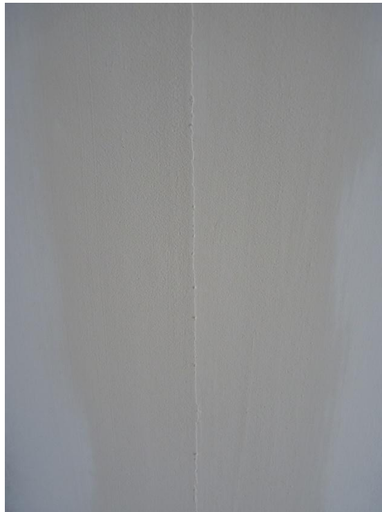
Photograph A.7. Plasterboard crack on the 2.4 m long wall on Side 2 formed after regime Long 5 (nominal 23 mm) taken after regime Long 5 (nominal 23 mm)
