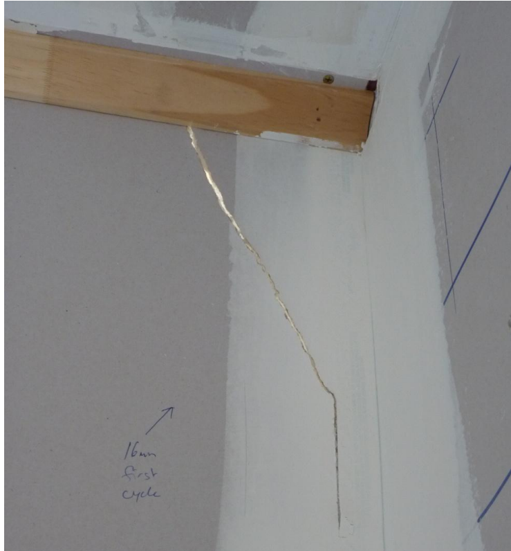
Photograph A.4. Plasterboard crack on the 3.6 m long wall on Side 2 formed after regime Long 4 (nominal 16 mm) taken after regime Long 5 (nominal 23 mm)
