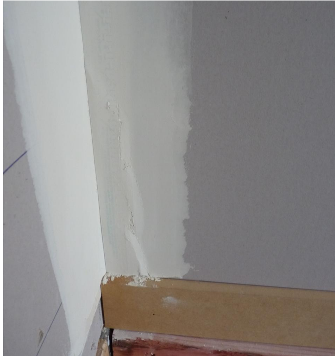
Photograph A.8. Plasterboard crack on the 2.4 m long wall on Side 2 formed after regime Long 4 (nominal 16 mm) taken after regime Long 5 (nominal 23 mm)
