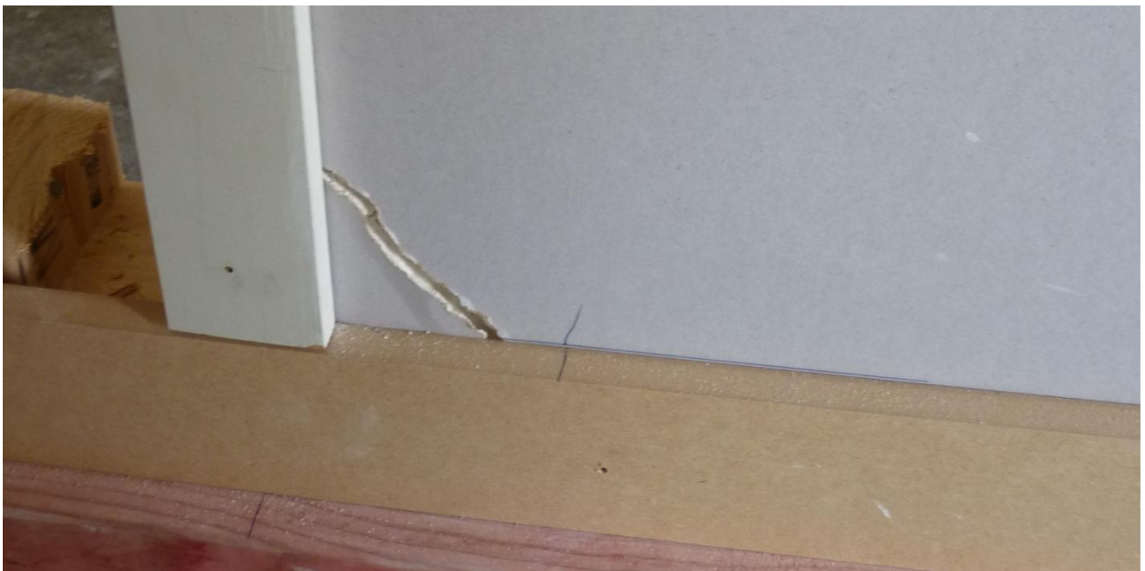
Photograph A.5. Plasterboard crack on the 3.6 m long wall on Side 2 formed after regime Long 3 (nominal 12 mm) taken after regime Long 5 (nominal 23 mm)
