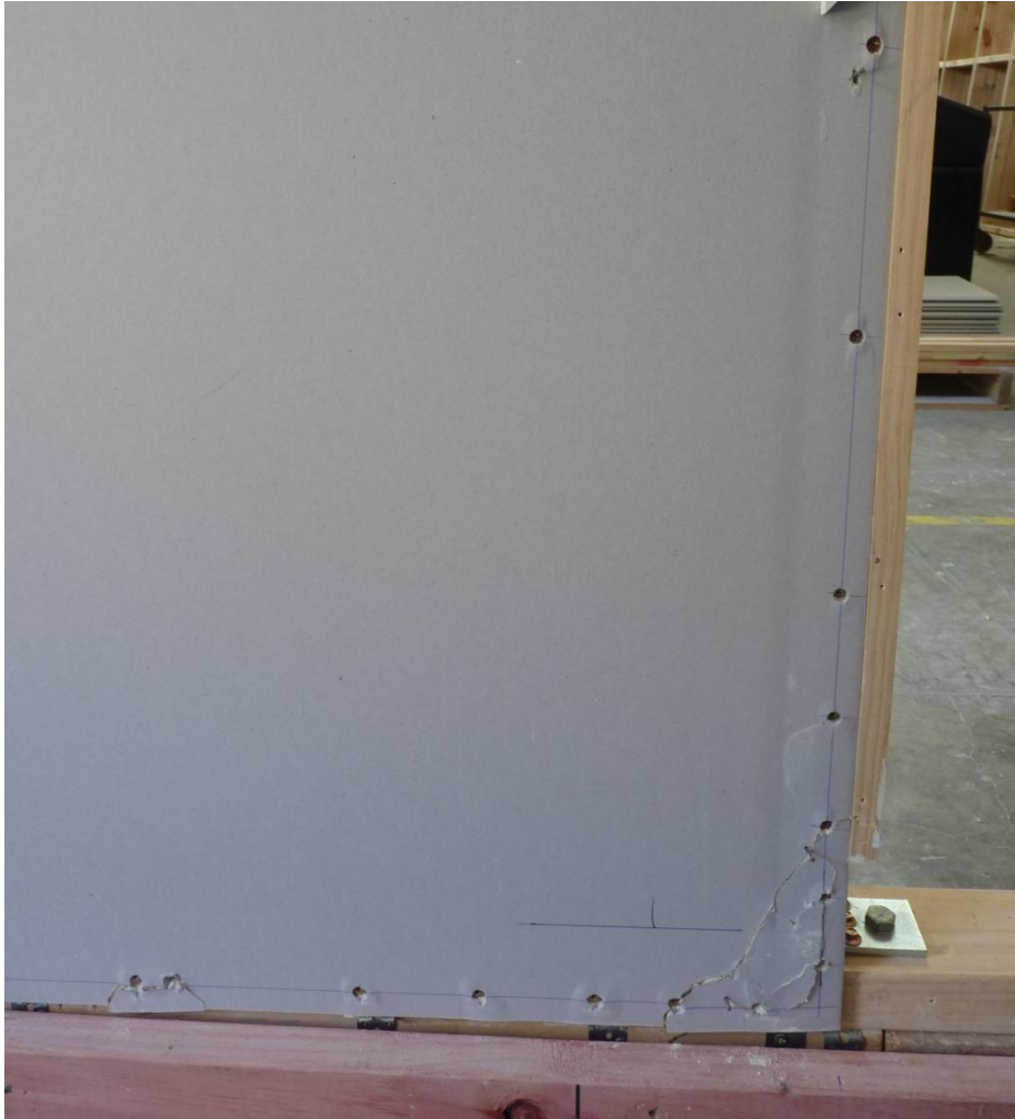
Photograph A.14. Plasterboard damage at the free end of the base of the 2.4 m long wall on Side 1 formed after regime Long 7 (nominal 45 mm)
