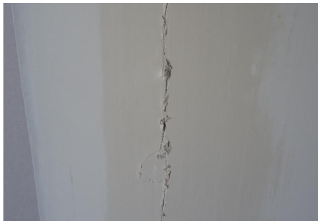
Photograph A.3. Plasterboard sheet joint crack on the 2.4 m long wall on Side 1 formed after regime Long 5 (nominal 23 mm) taken after regime Long 5 (nominal 23 mm)
