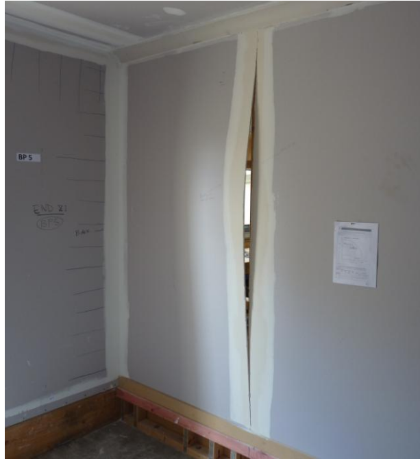
Photograph A.12. Plasterboard joint tear on the 2.4 m long wall on Side 1 formed after regime Long 6 (nominal 32 mm) taken after regime Long 6 (nominal 32 mm)
