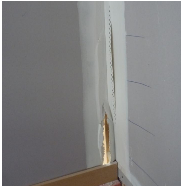
Photograph A.9. Plasterboard crack on the 3.6 m long wall on Side 1 formed after regime Long 6 (nominal 32 mm) taken after regime Long 6 (nominal 32 mm)
