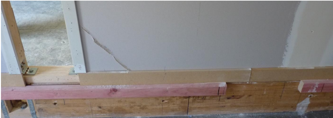
Photograph A.1. Plasterboard crack on the 3.6 m long wall on Side 1 formed after regime Long 3 (nominal 12 mm) taken after regime Long 5 (nominal 23 mm)
