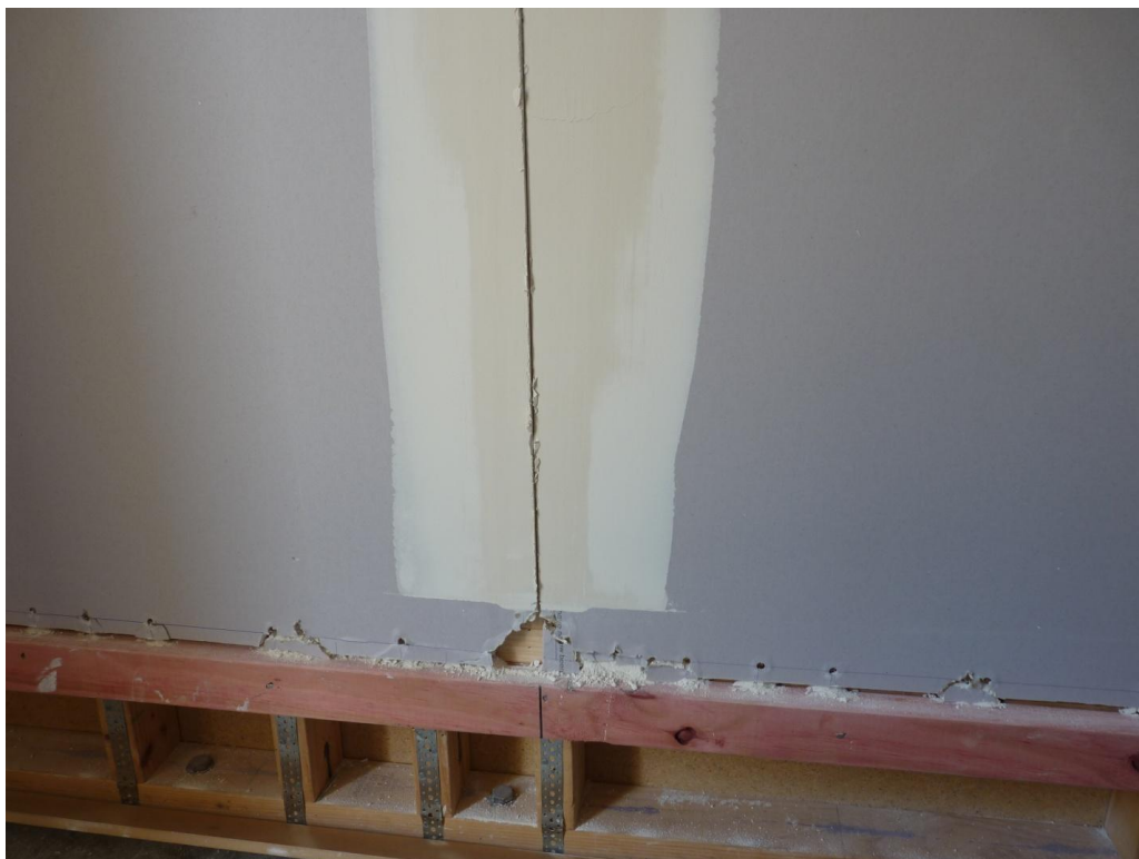
Photograph A.13. Plasterboard sheet damage at the mid-length of the base of the 2.4 m long wall on Side 1 formed after regime Long 7 (nominal 45 mm). Note that the skirting has been removed to show damage to bottom sheet fixings
