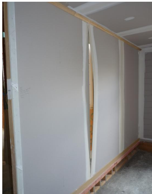
Photograph A.11. Plasterboard joint tear on the 3.6 m long wall on Side 1 formed after regime Long 6 (nominal 32 mm) taken after regime Long 6 (nominal 32 mm)
