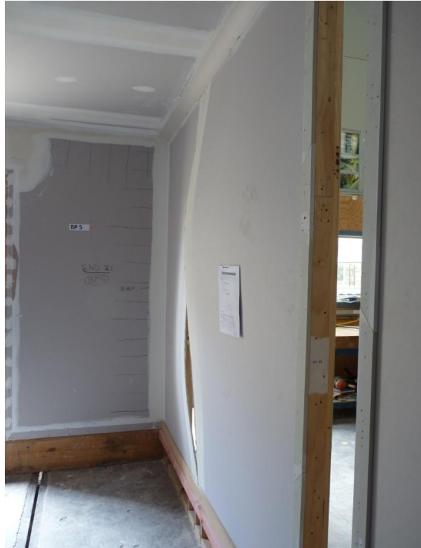
Photograph A.10. Plasterboard joint tear on the 3.6 m long wall on Side 1 formed after regime Long 6 (nominal 32 mm) taken after regime Long 6 (nominal 32 mm)
