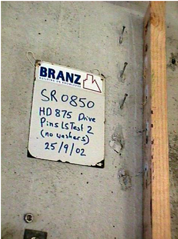
Photograph 6. Failure mode E (note, the lower 2 pins show failure mode D)
