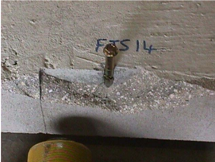
Photograph 2. Failure mode A
