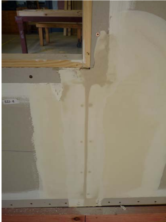
Photograph D17 of another vertical crack repaired after Phase 3
