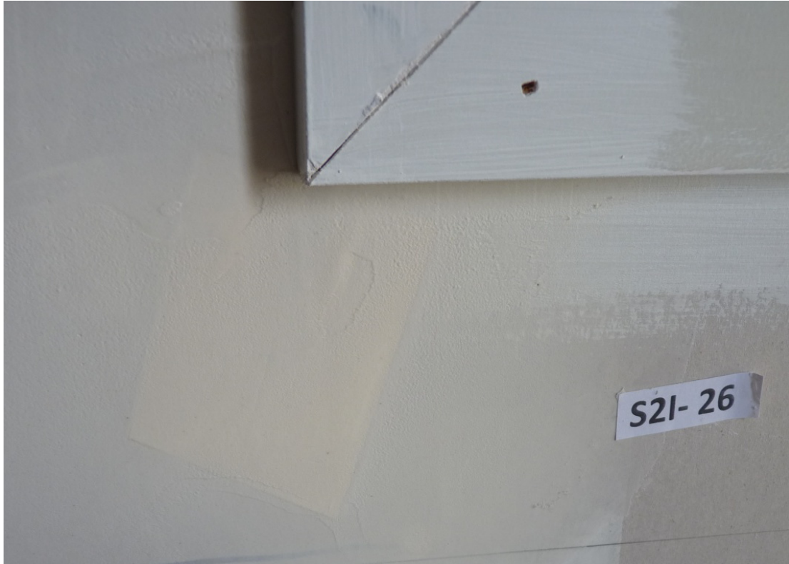
Photograph D7 cosmetic repair after Phase 1. Repaired diagonal crack before final plaster finish
