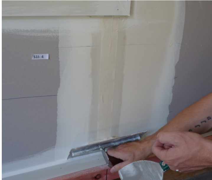
Photograph D11 cosmetic repair after Phase 1. Vertical crack gouged out and paper tape added
