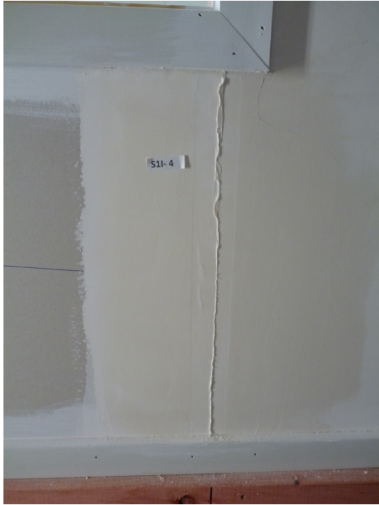
Photograph D13 taken after test P2D16. Vertical plasterboard cracks had increased in severity
