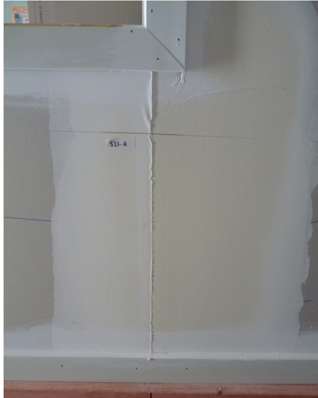
Photograph D3 taken after test P1D12. Typical plasterboard crack along plasterboard joints constructed at opening corners
