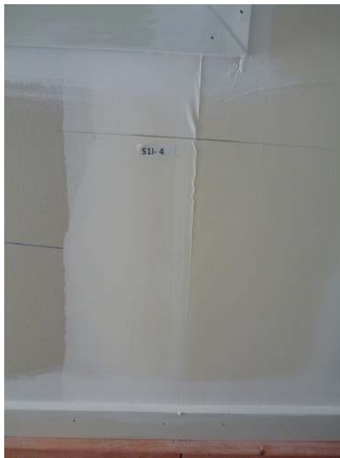
Photograph D2 taken after test P1D8. Typical plasterboard crack and ridge line which formed along most plasterboard joints constructed at opening corners
