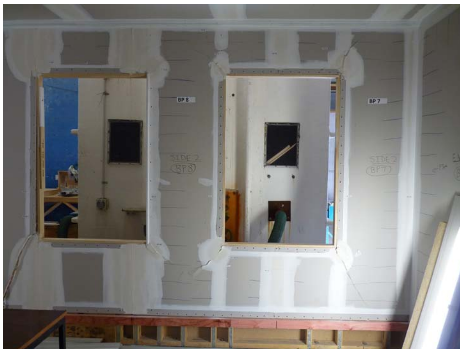
Photograph D22 taken after test P4D40 showing diagonal cracks from both the J_NOT_Openings and J@Openings joints
