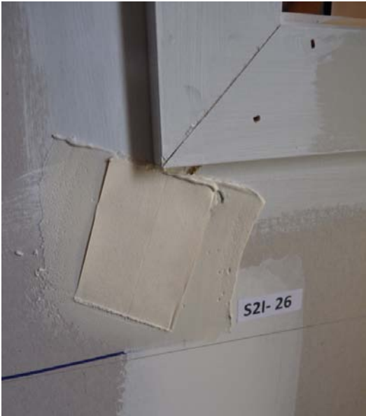
Photograph D6 cosmetic repair after Phase 1. Plaster coating and adding paper reinforcing
