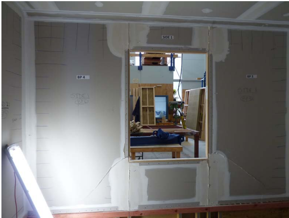
Photograph D21 taken after test P4D40. Note that diagonal cracks had formed at both the J_NOT_OPENINGS and J@Openings joints
