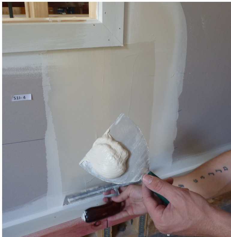
Photograph D12 cosmetic repair after Phase 1. Before final coat over vertical crack
