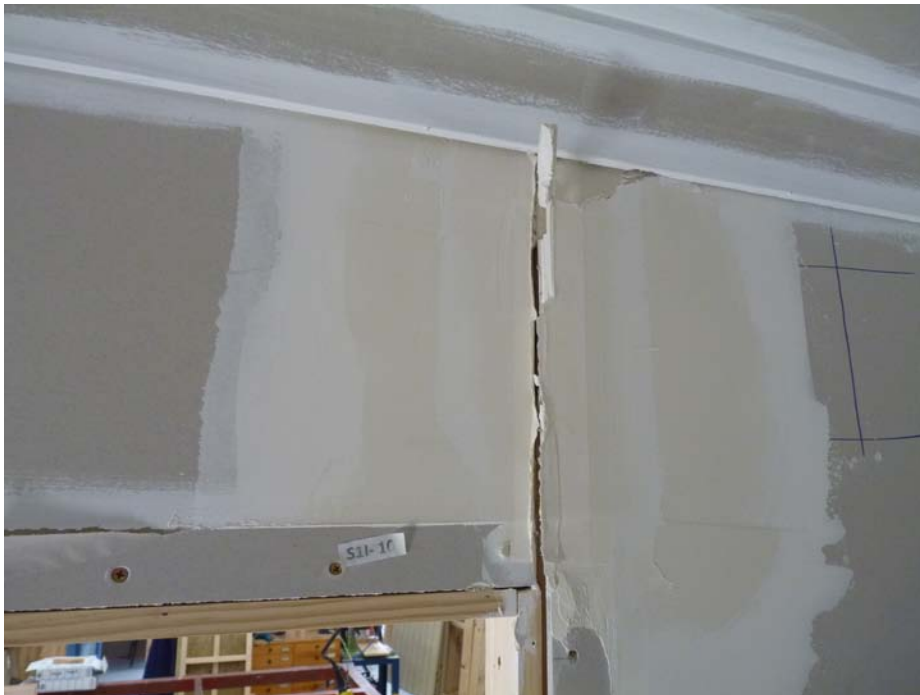
Photograph D20 taken after test P4D40. Vertical crack widths had increased in width and some sheets had become loose
