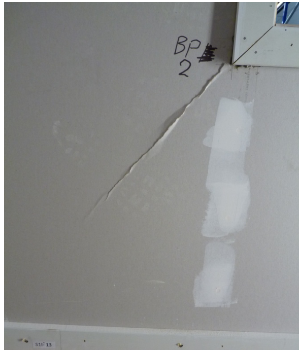
Photograph D24 taken after test P5D16. Crack length = 550 mm
