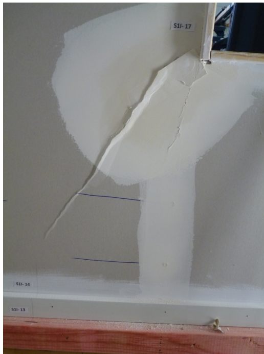
Photograph D14 taken after test P2D16. The largest of the diagonal cracks had now increased in length
