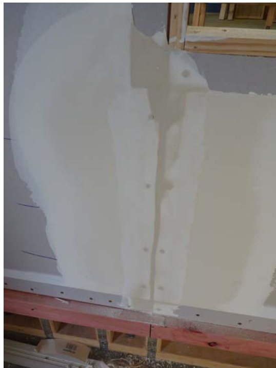
Photograph D16 of the crack repaired in Photograph D15
