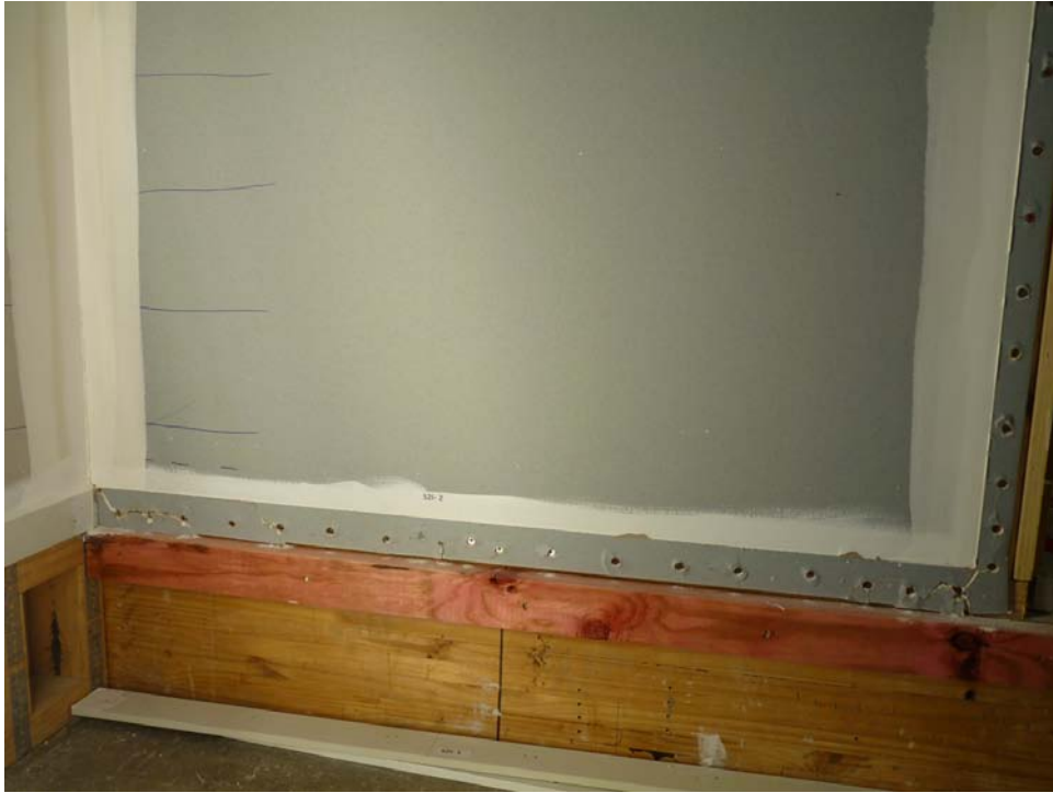
Photograph D23 taken after test P4D40. Plasterboard distress at screw locations
