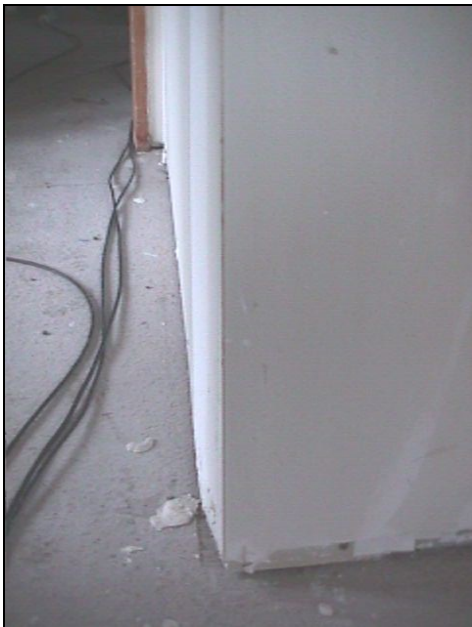
Figure 20: View showing misalignment of the plate in the orthogonal wall
