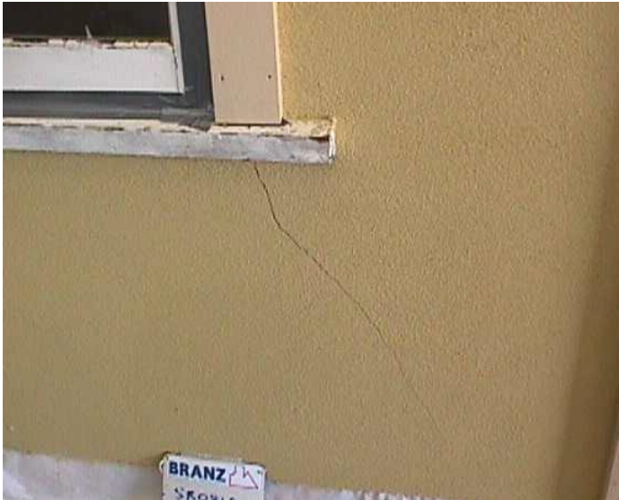
Figure 35: Diagonal cracks in the fibre-cement wall from the bottom corners of the window
