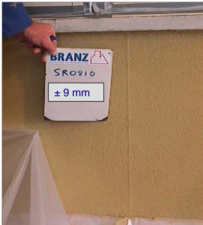
Figure 28: Bulge in fibre-cement cladding joint after \pm 9 mm racking
