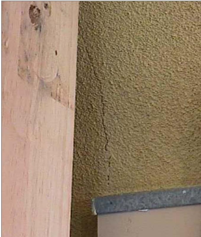
Figure 29: 1 mm wide crack in fibre-cement cladding above window head
