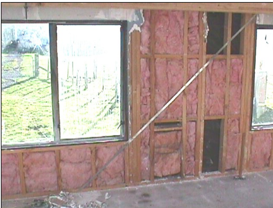
Figure 17: Light steel strap brace (was fixed to Wall 1 while pulled to a position beyond vertical)
