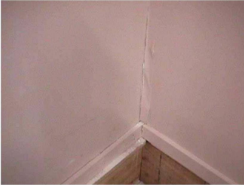
Figure 11: Wrinkling and crumbling of the plasterboard at the painted corner
