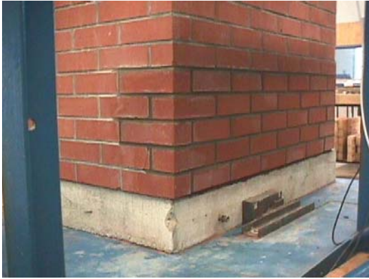
Figure 6: Veneer repair completed (note mortar is darker because it is still fresh)
