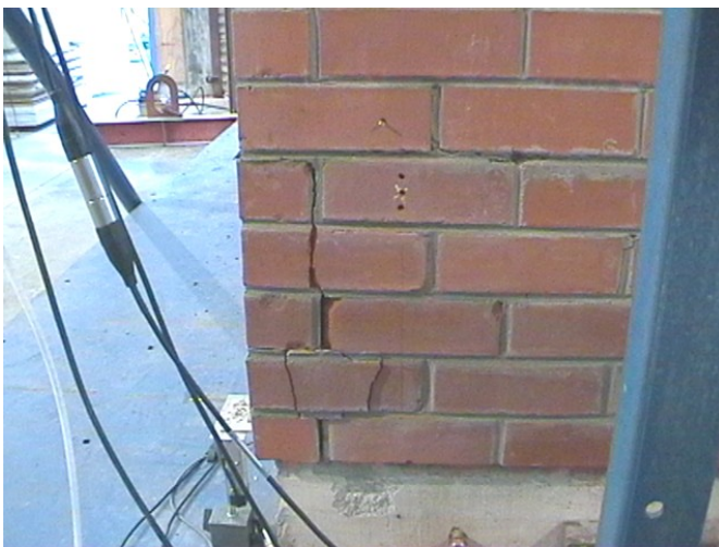
Figure 8: View of damage to repaired veneer in the return corner
