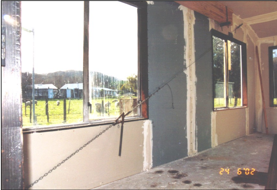
Figure 16: Wire fence strainer used to try to re-align the wall
