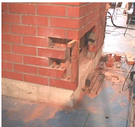
Figure 4: Damaged corner removed and propped
