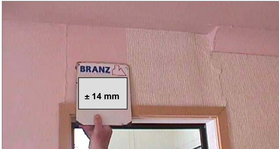
Figure 31: Damage to the interior surfaces at the joints between sheets
