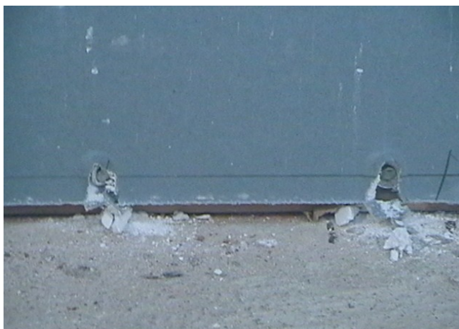
Figure 3: Evidence of nails pulling through the edge of the plasterboard sheets
