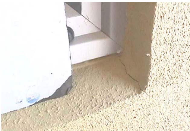
Figure 30: Crack in the corner of the EIFS cladding at the corner of the window
