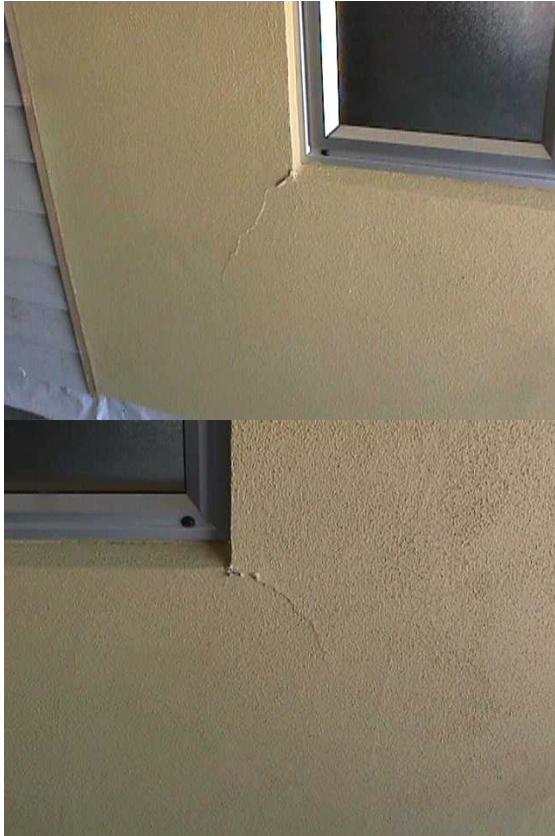
Figure 32: Cracking damage in EIFS cladding after cycles to \pm 24 mm
