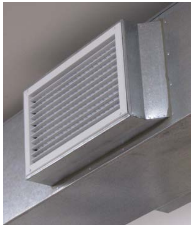
Cleaning access for ducts.
