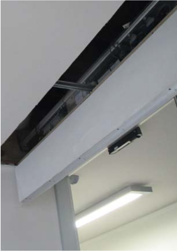
Retrofitted panel to allow access to automatic door motor.
