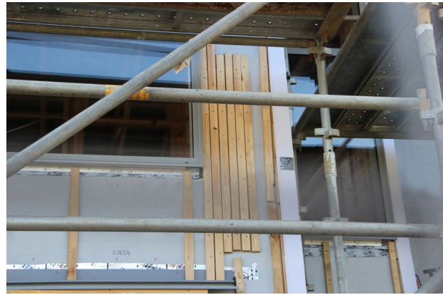
An excessive number of battens that will impact drainage and drying in the wall cavity.
