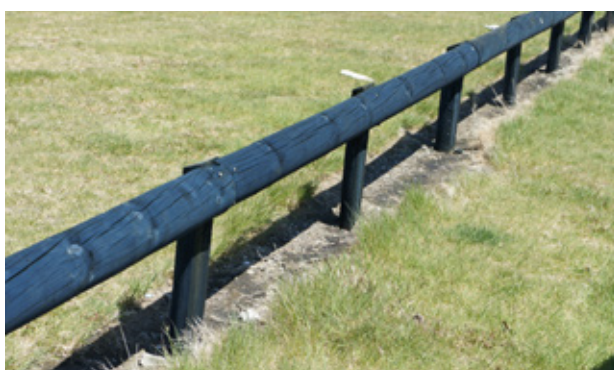
Figure 10. Wood discolouration in an area with strong geothermal influences.
