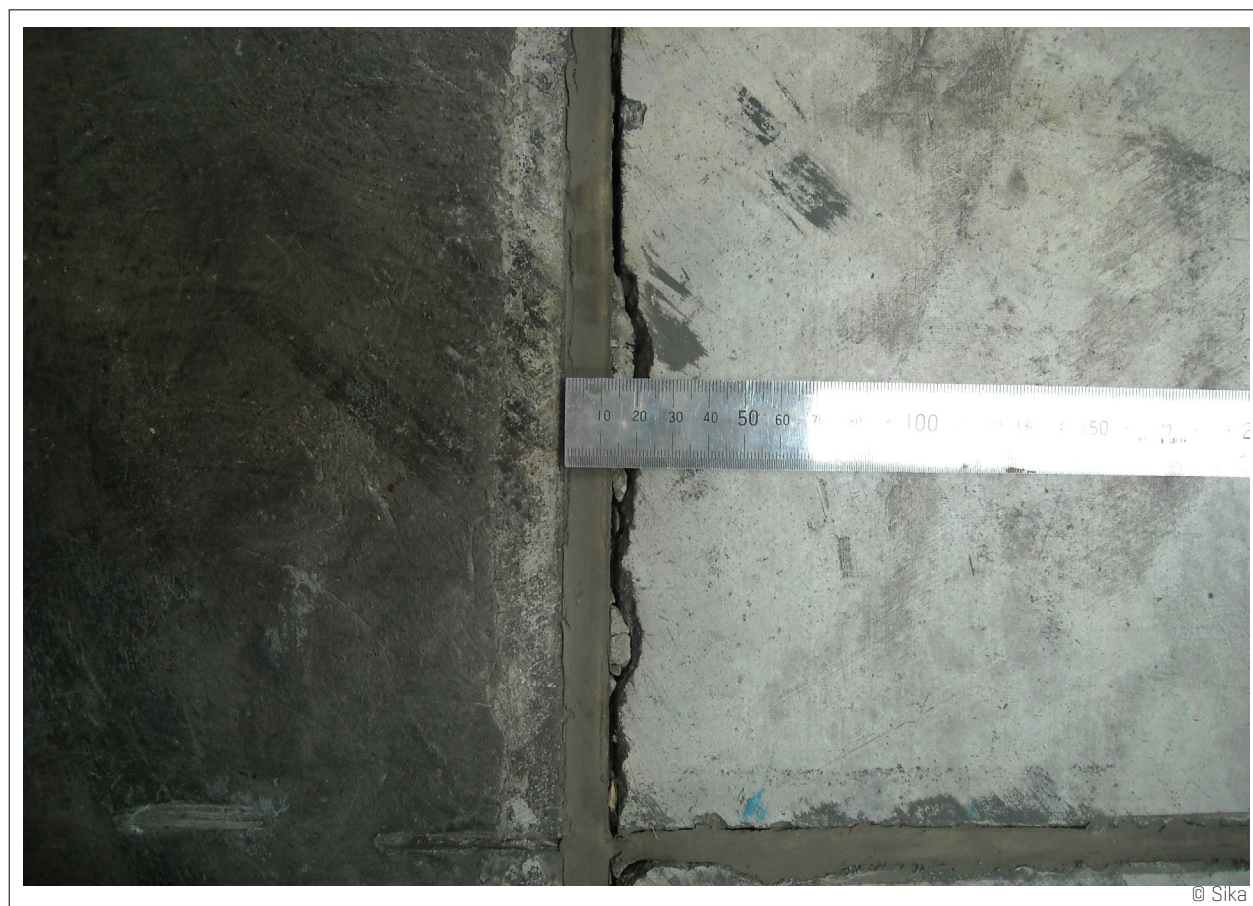
Adhesive sealant failure [loss of edge bond].
