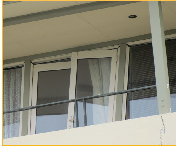
Damage resulting from differential movement between the floor structure and the roof structure.
