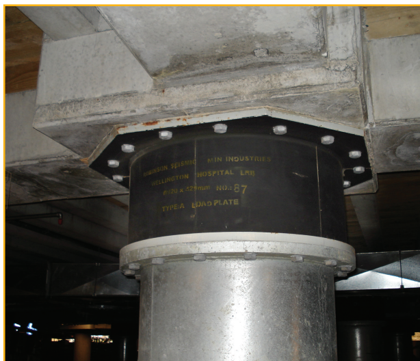
Base isolator, Wellington Hospital.
