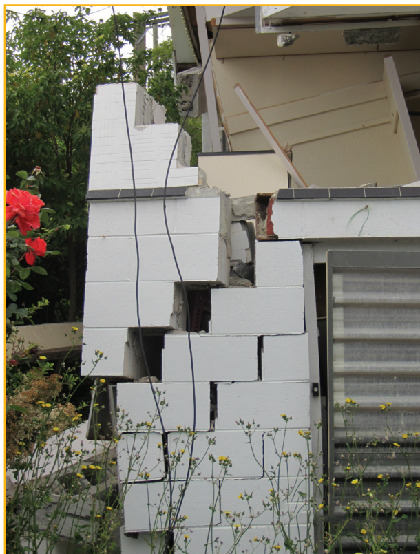
Unreinforced masonry damage.
