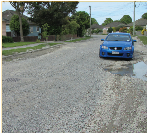
Road damage caused by liquefaction.
