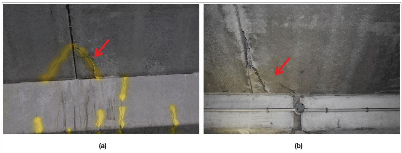
Figure 11: (a) corner crack with grout seeping out observed in the building investigated (b) corner crack observed in a carpark in Auckland
