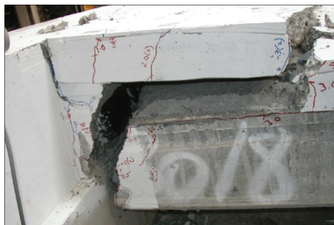
Figure 1 Steep positive moment crack along the ledge of the seating resulted in floor collapse (Bull and Matthews 2003)
