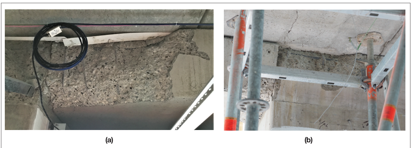
Figure 9: Significant support ledge spalling observed at different locations in the building (a) Pier 3 level 1 (modified from Siddiqui et al. (2019a)) (b) Pier 2 level 1
