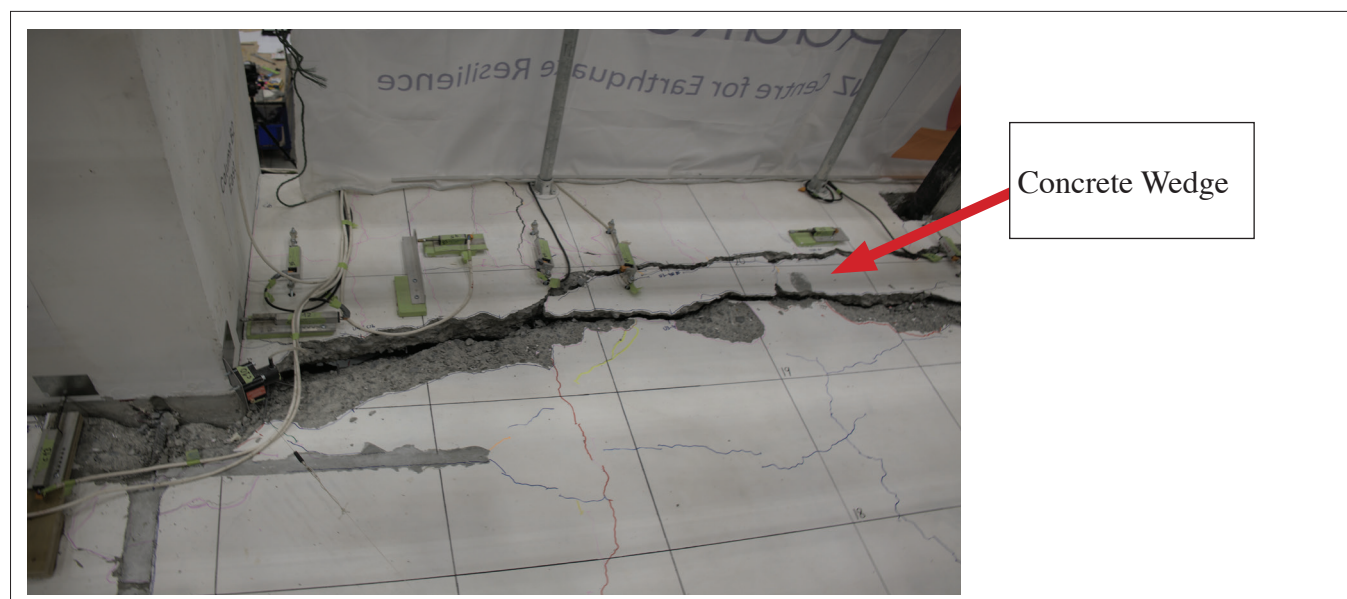
Figure 21: Beam-unit crack interface concrete wedge on east side of column B2 at 4.0% drift
