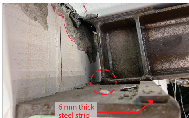
Figure 14: Front end of strongback in contact with the seating angle (first observed at 3% inter-storey drift).
