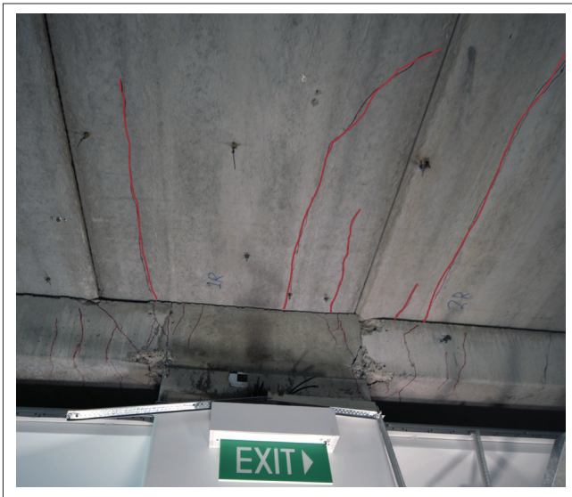
Figure 12: longitudinal cracking of HC unit soffit
