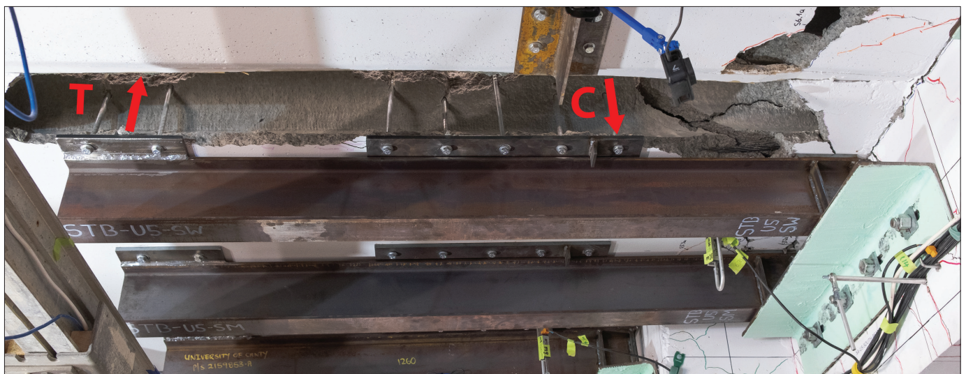
Figure 11: Strongback retrofit carrying the load of the floor after a negative moment failure has occurred. (Photo taken at 5% inter-storey drift)
