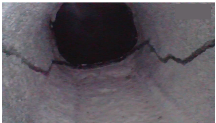
(b) Internal cracking at a shallow angle (Büker et al. 2021)
