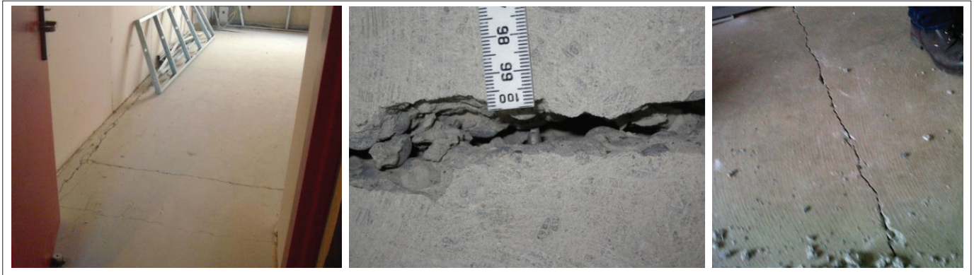
Figure 3: Cracking between individual precast concrete flooring units and mesh rupture observed following the 2011 Christchurch earthquakes (Henry and Ingham 2012)
