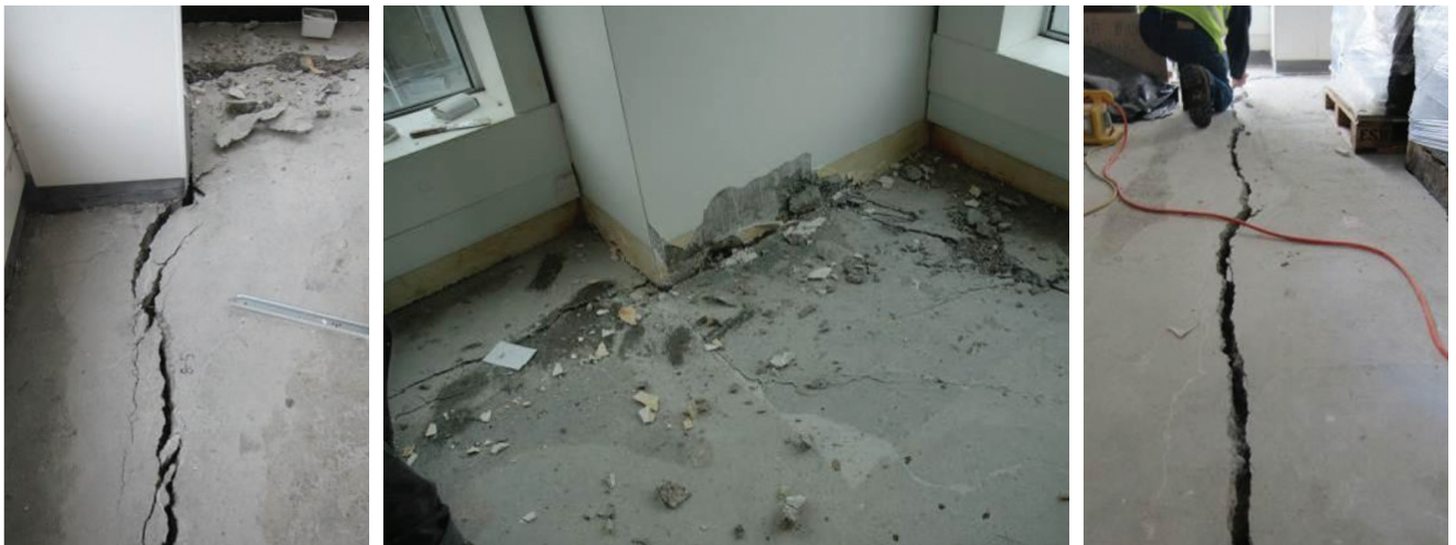
(a) Significant floor perimeter cracking following the 2011 Christchurch earthquakes (Kam et al. 2011)
