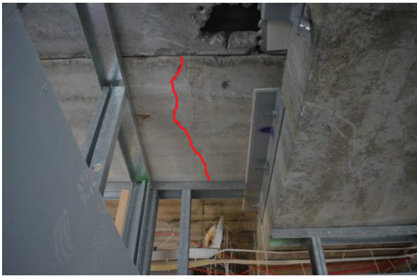
(a) Transverse soffit cracking away from the support and seating angle (Henry et al. 2017)
