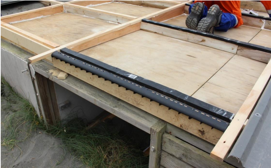
Figure 3. Over-fascia vent next to a vented batten, terminating the lower end of the roof cavity.
