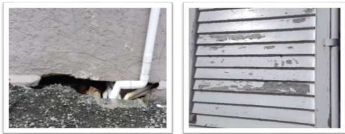
Figure 14. Wall cladding was in poor or serious condition for one in five dwellings.
