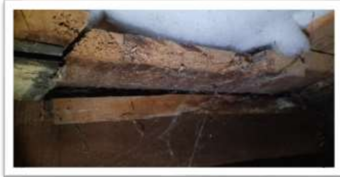
Figure 23. Signs of borer in subfloor timber.
