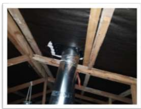
Figure 28. Damaged roof underlay.
