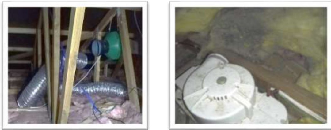
Figure 38. Mechanical extract ventilation must extract outside not to the roof space.
