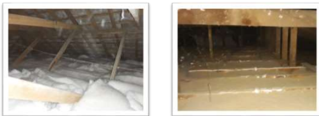
Figure 30. Roof spaces should be insulated to help prevent heat loss from the home. Around half of houses surveyed lacked adequate insulation in the roof.
