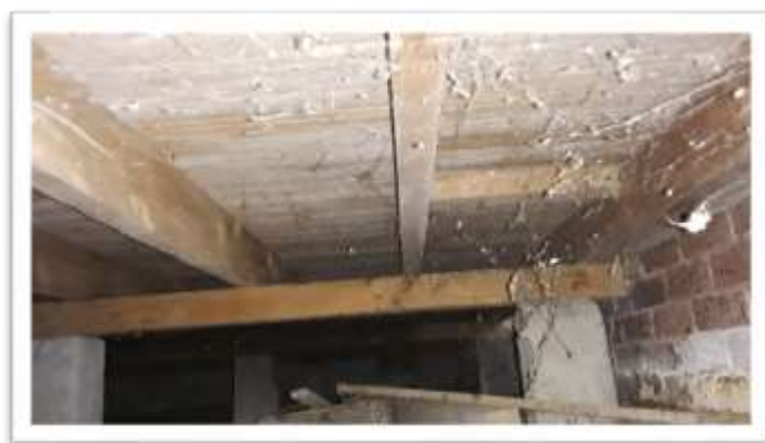
Figure 34. Almost one-quarter of houses with a subfloor cavity lacked adequate insulation. This applied to owned and rented dwellings.
