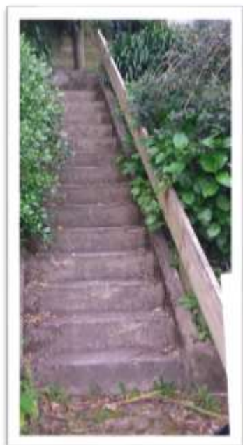
Figure 50. Overgrown vegetation can pose an access hazard.
