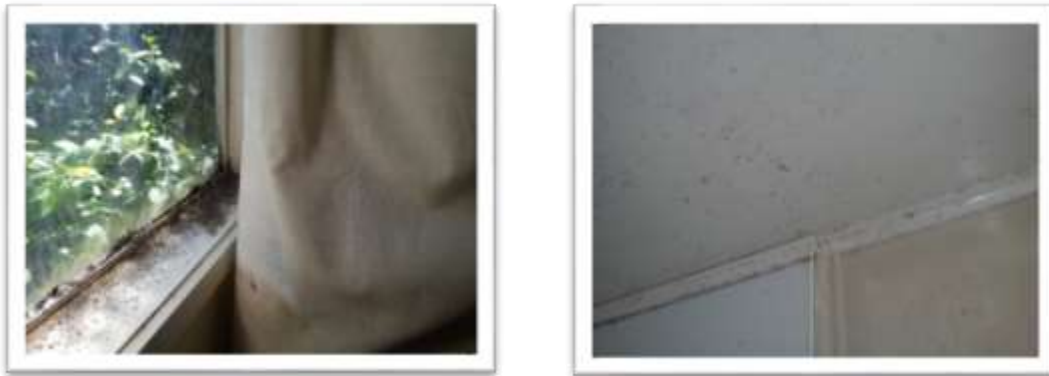
Figure 25. An assessment of visible mould was applied to all surfaces, including wall, floor and ceiling linings, windows and curtains.
