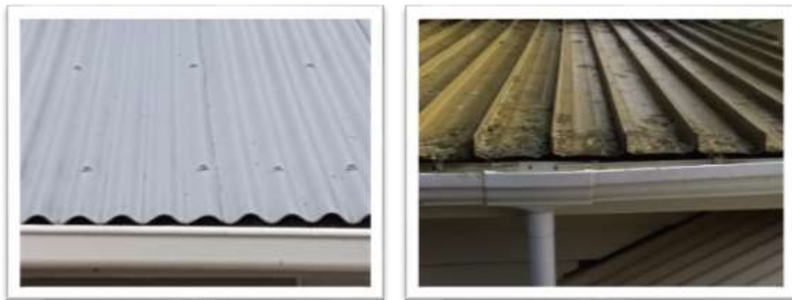
Figure 12. Almost half of roofs were in excellent or good condition, and one in 10 roofs were considered to be in poor or serious condition.
