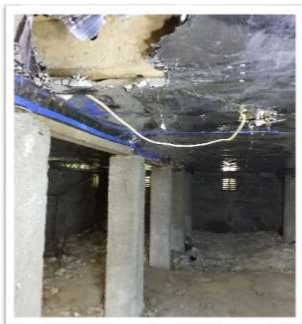
Figure 32. Subfloor foil insulation is prone to damage
