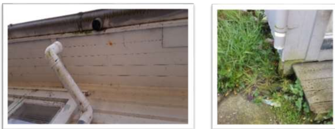
Figure 21. One-third of dwellings required some maintenance or repair to guttering or downpipes.
