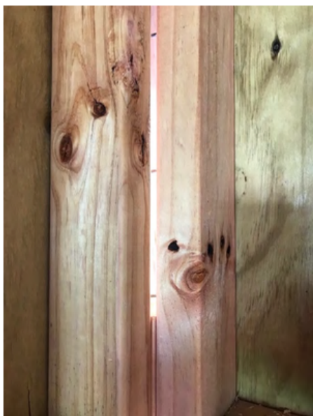
An external corner junction showing the light coming through the wall underlay. Installing insulation in the gap between the studs is practically impossible at this stage with the underlay in place.
