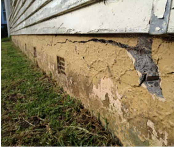
Figure 11: Ring foundation damage requiring significant repairs
