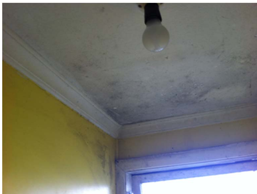
Figure 6: Mould noted in one of the houses
