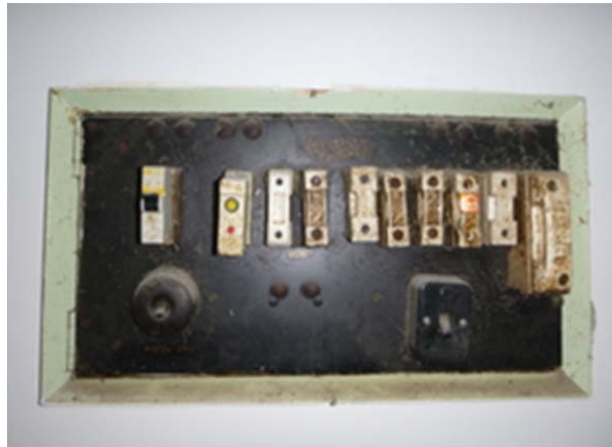
Figure 43: A circuit board requiring replacement
