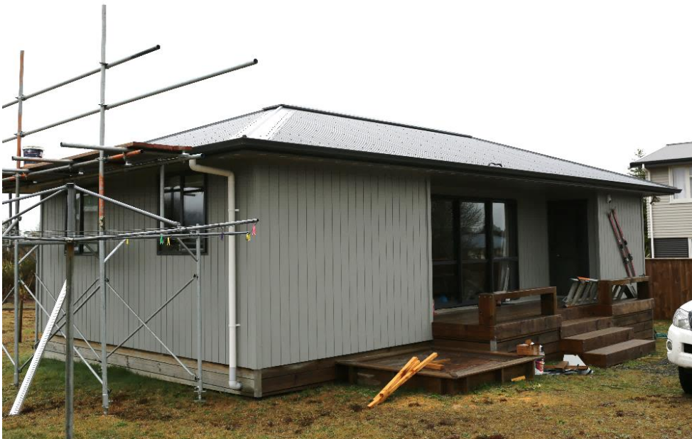
Figure 1. Residential building with standard gable roof construction used for airflow resistance measurements. The entrance side of the house shown here is oriented towards the north.
