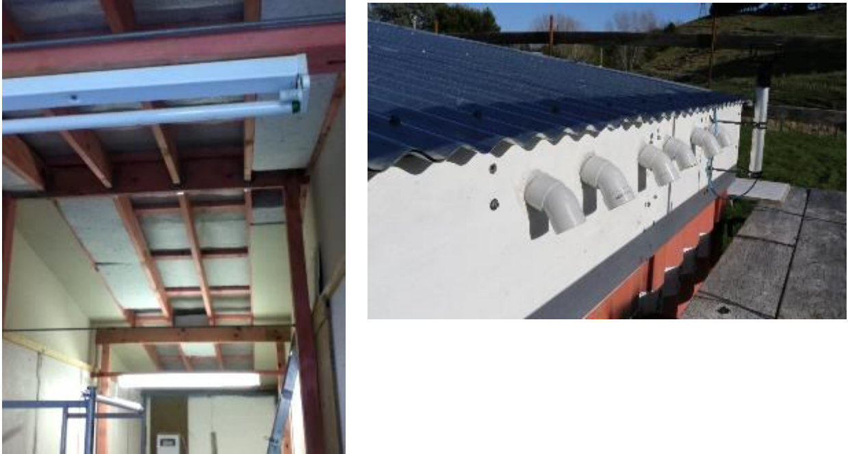
Figure 12. Skillion-type roof with some of the ceiling panels removed (left). Ventilation channels were added at the northern and southern eaves (right)
