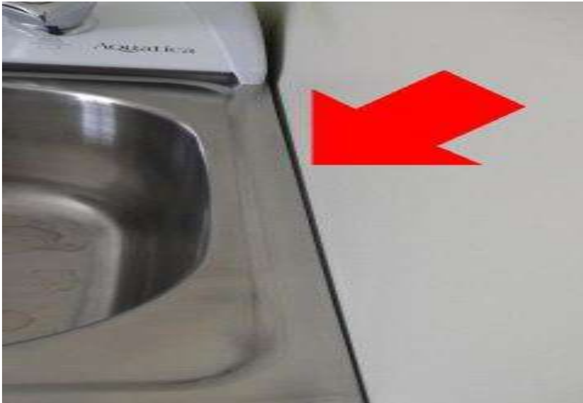
No seal at sink-wall junction.
