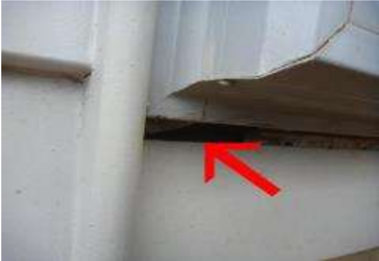
Gaps between the window frame and the cladding
