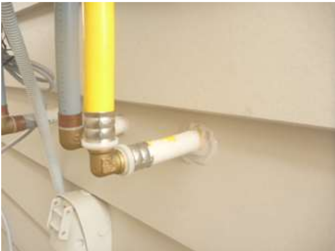
Sealant around penetrations should have an escutcheon to protect the sealant.
