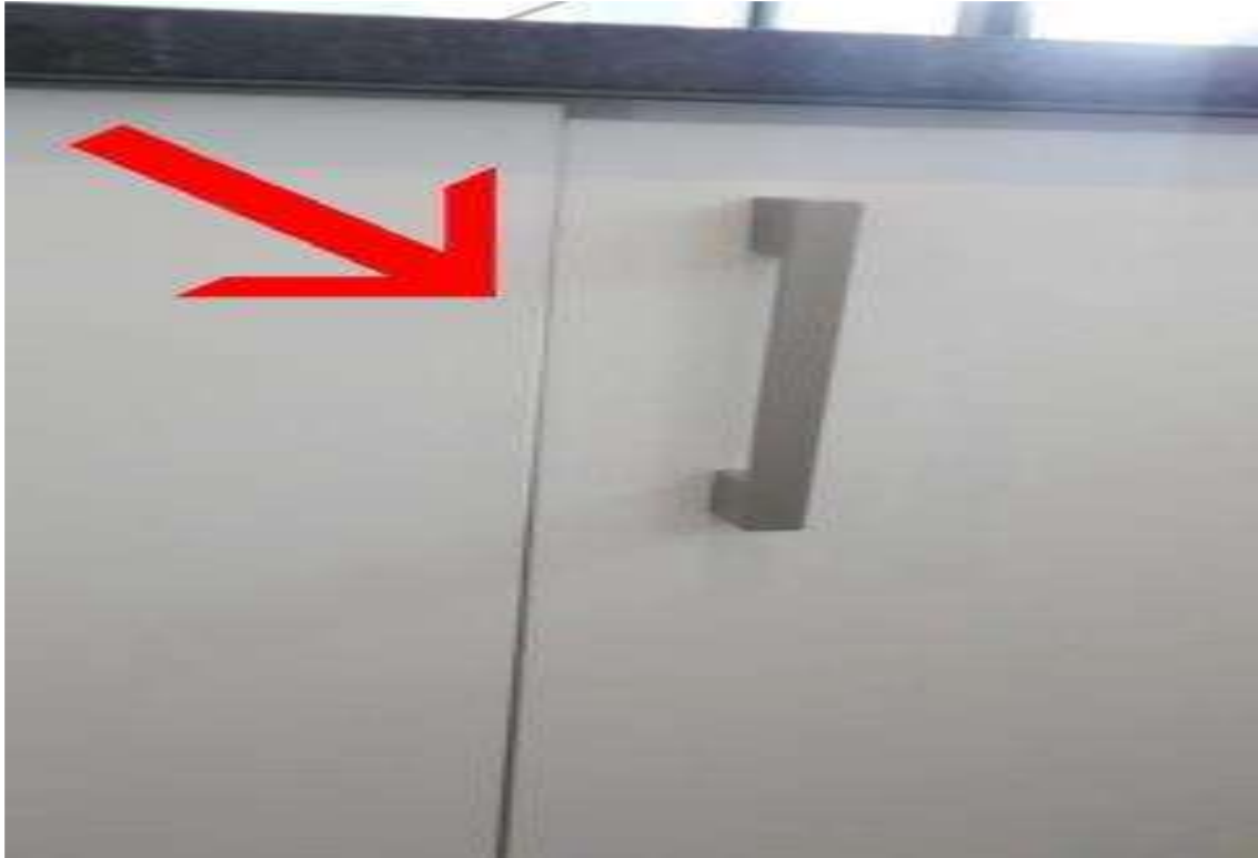
Ill-fitting cupboard door
