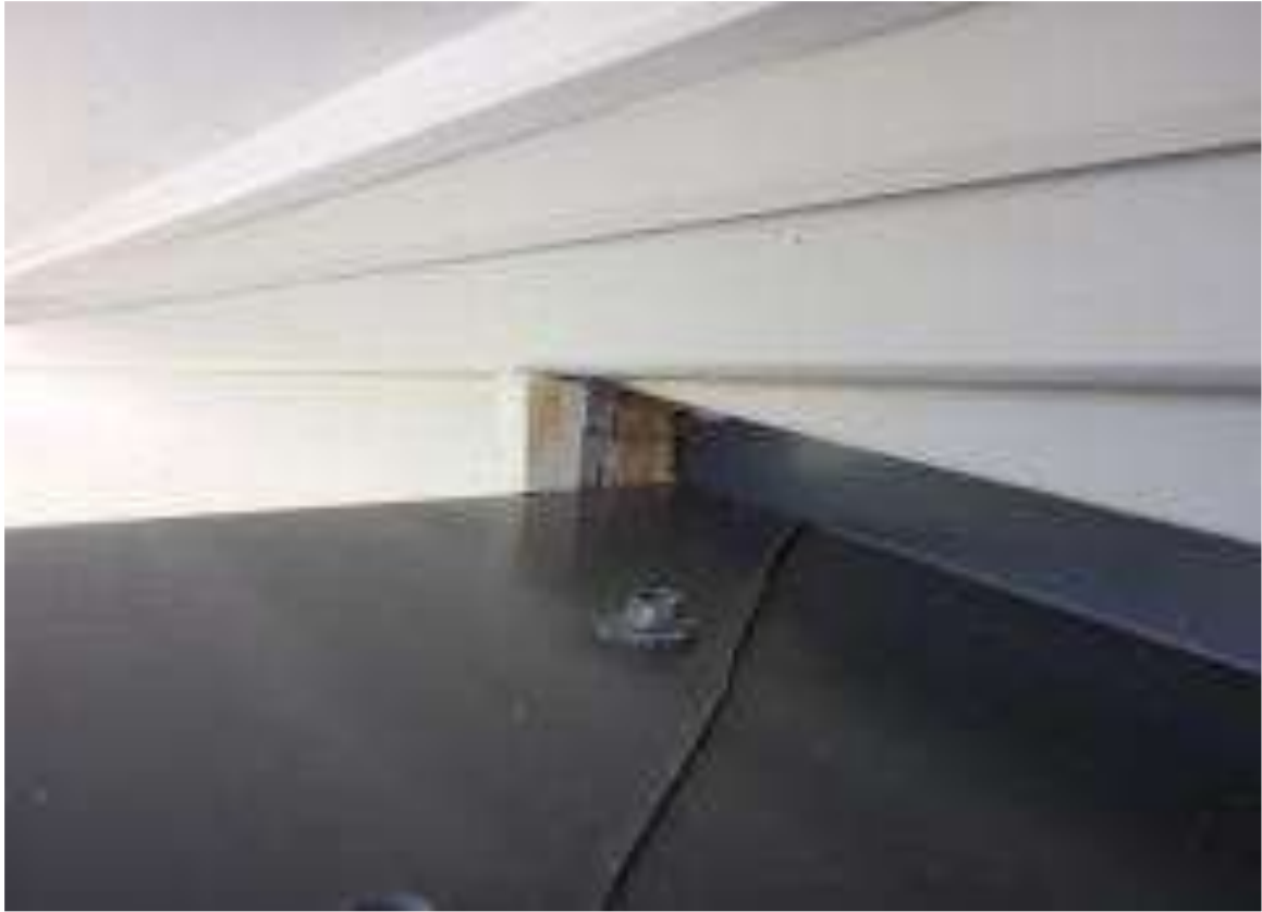
Apron flashing incomplete at corner with exposed timber.
