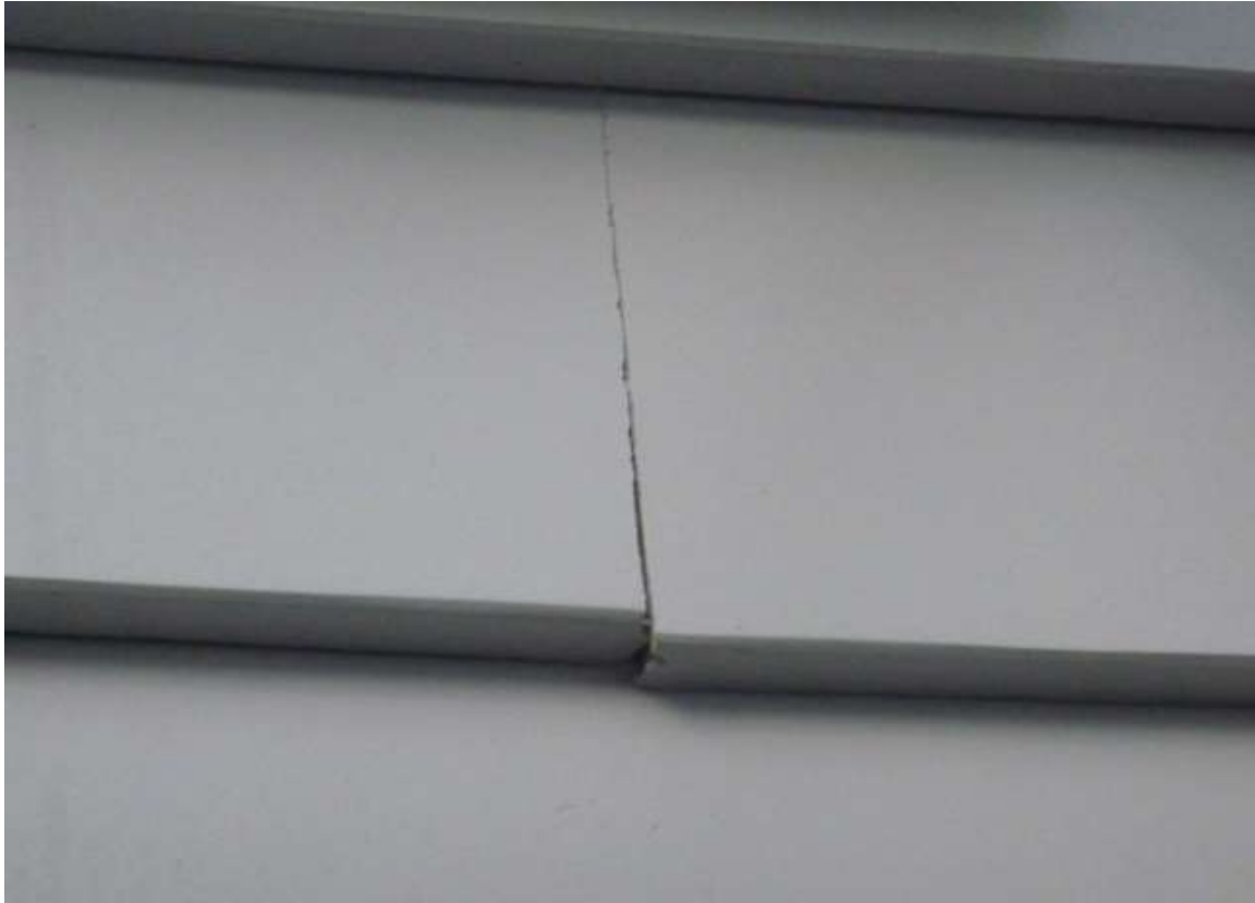
Poor weatherboard junction potentially allowing moisture penetration.
