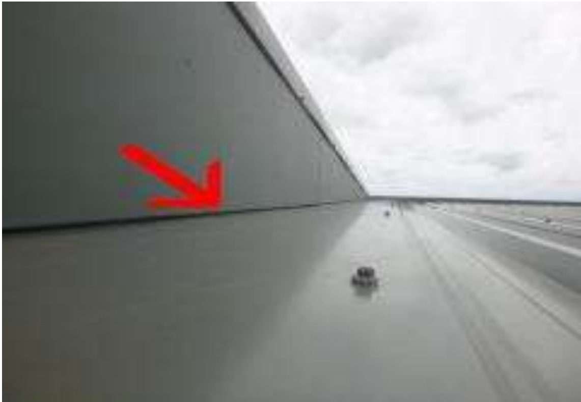
Inadequate clearance between the cladding and to the apron flashing
