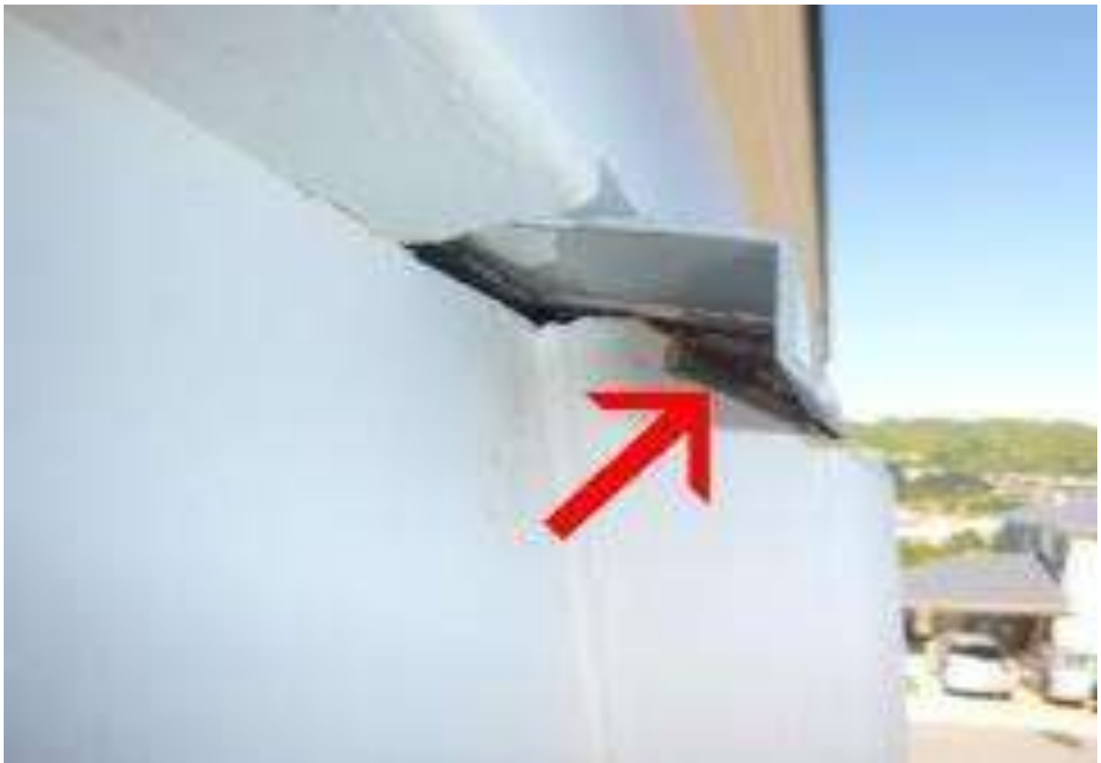
Head flashing does not cover scribe, unpainted and poorly cut scribe.
