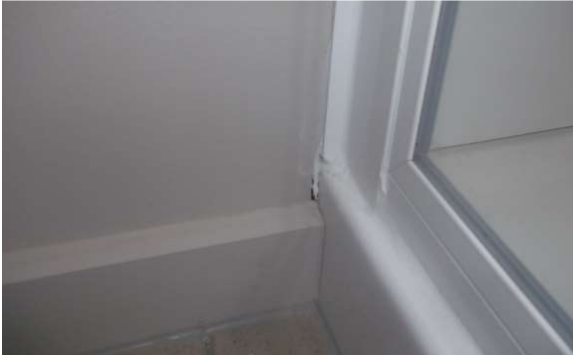
Poor sealing between the shower frame and the plasterboard.
