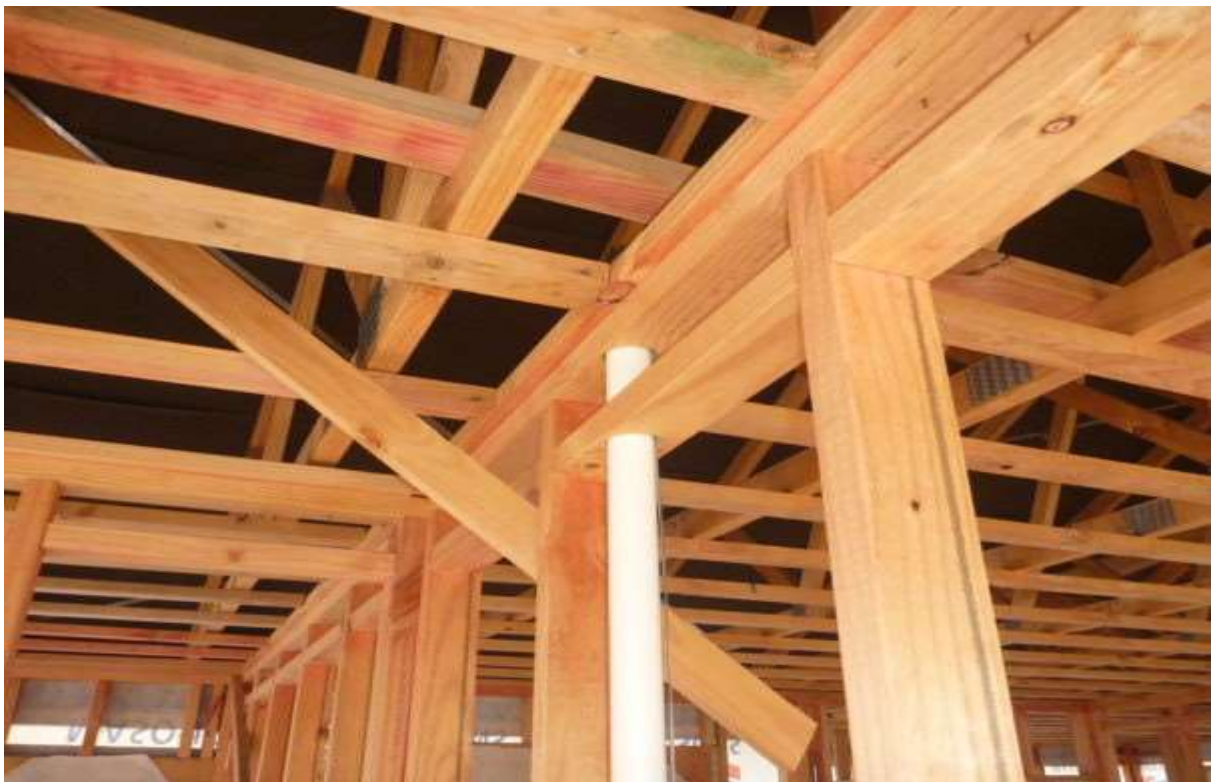
Un-reinforced top plate cut-out.
