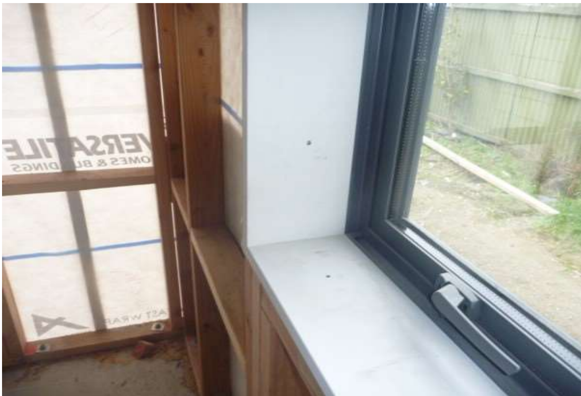
Inadequate fixing of window jamb to framing
