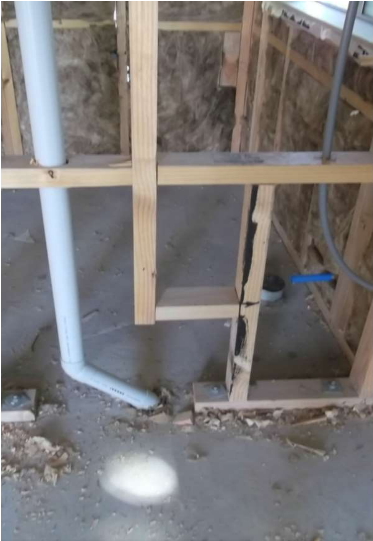
A large cut-out which the builder said would be repaired (but repairs are unlikely to be adequate due to the geometry). Appears to be a bracing wall re HD bolts.
