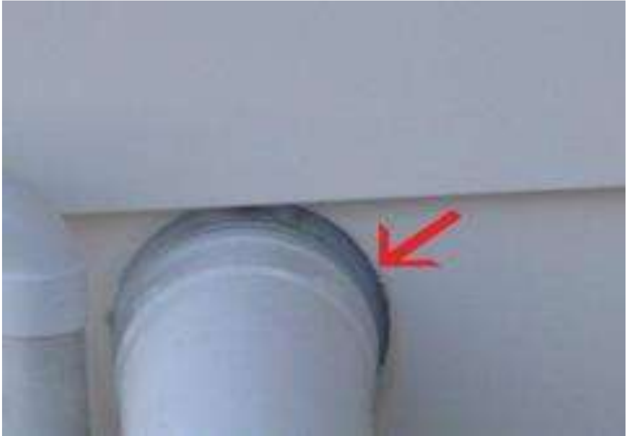
No sealing of the pipe cladding penetration.
