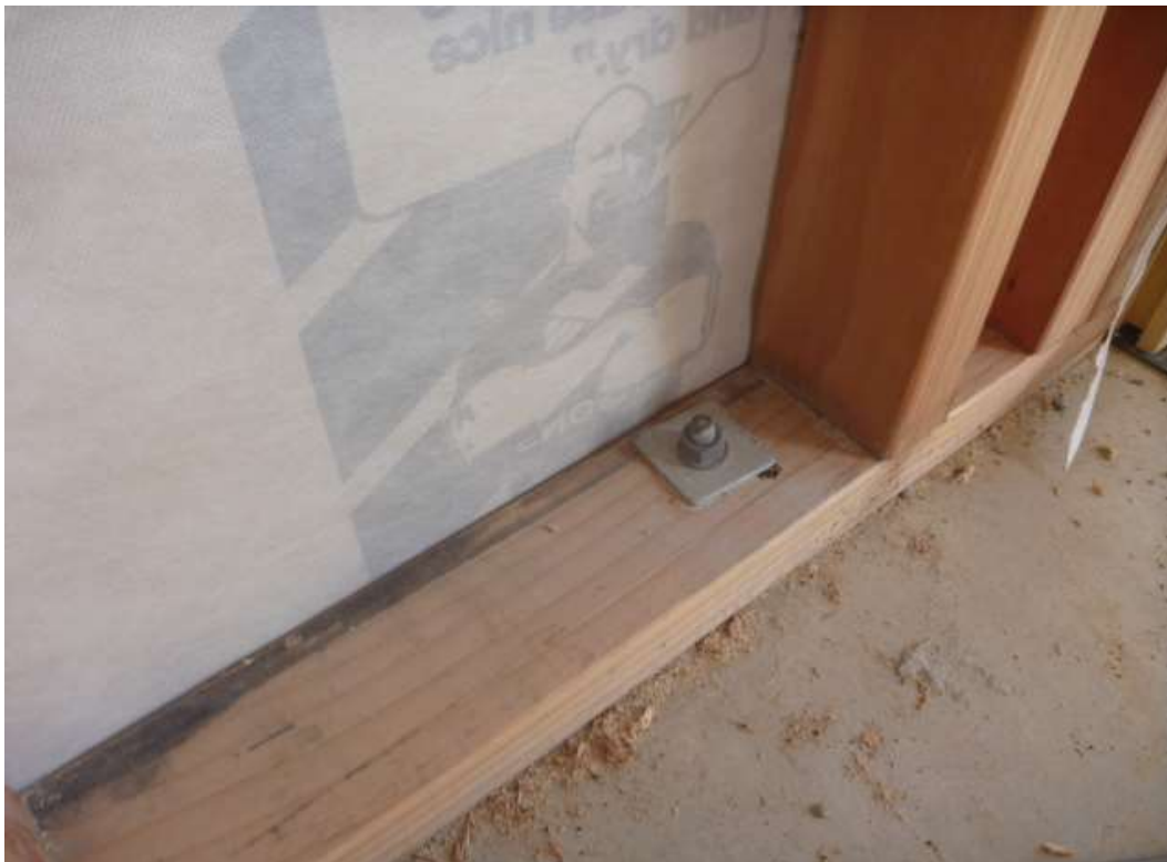
Holding down bolt is too close to the edge of the slab.
