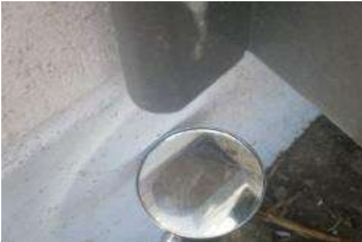
Underside of scribe is not painted.
