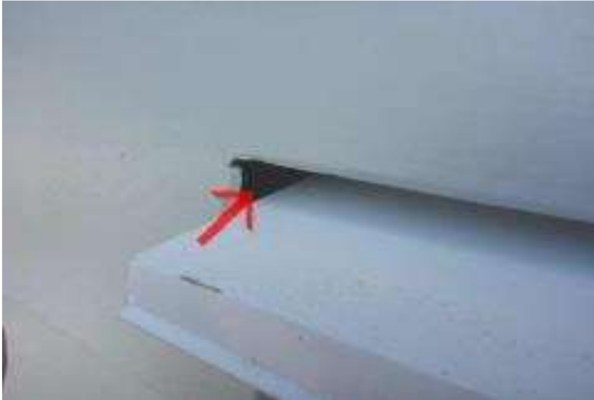
No stop-end on head flashing
