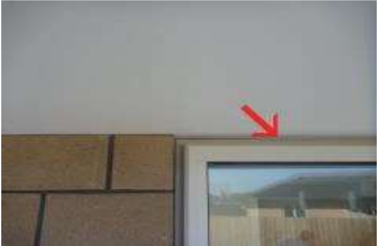
No bead between soffit and window frame
