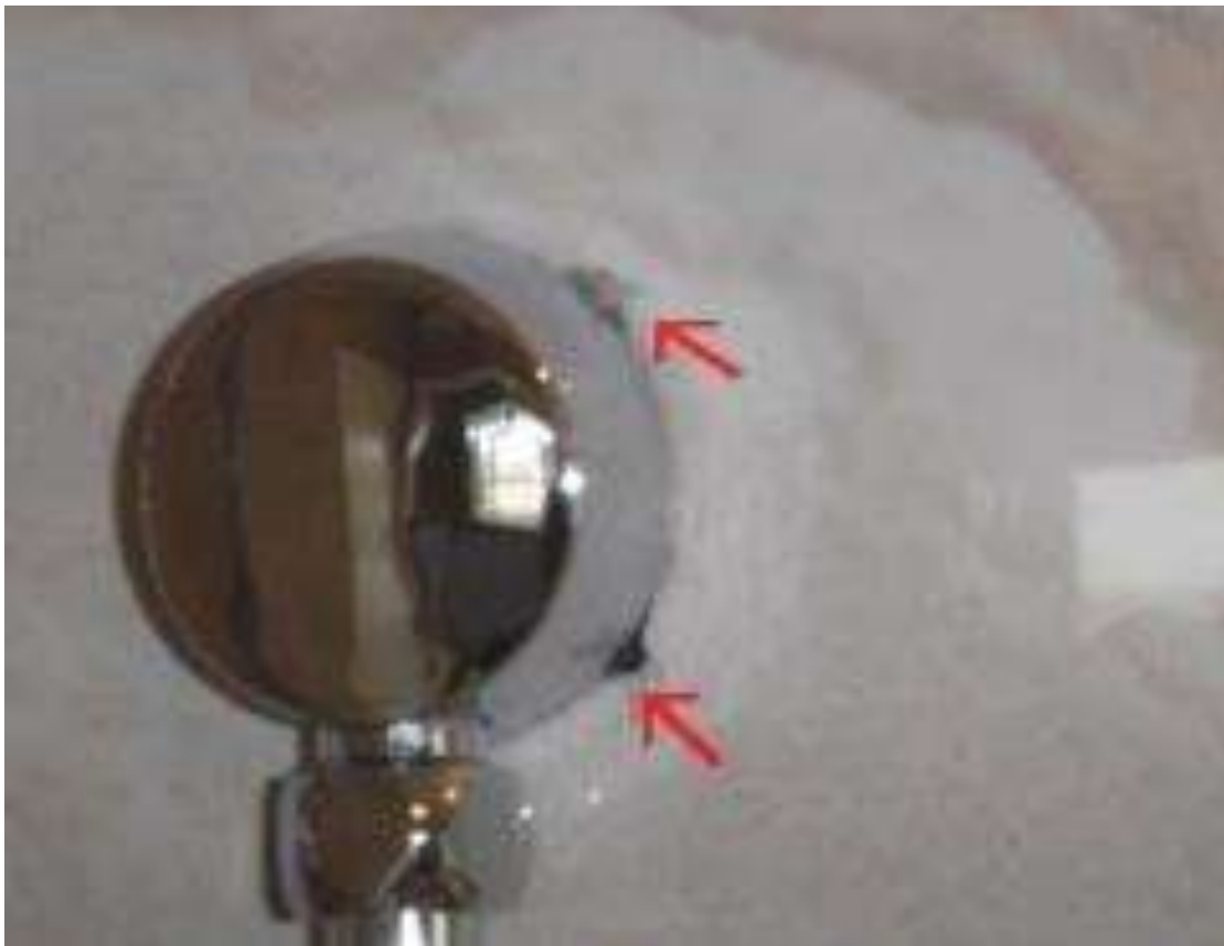
Shower lining with gaps around the pipe inlet
