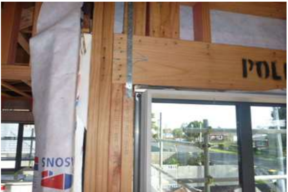
Lintel strap is incorrectly positioned.
