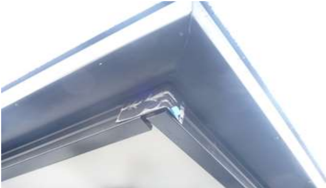
Untidy workmanship at the fascia junction.
