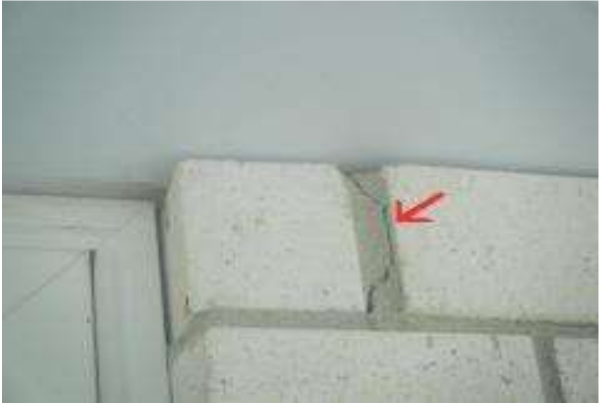
Loose clay brick.
