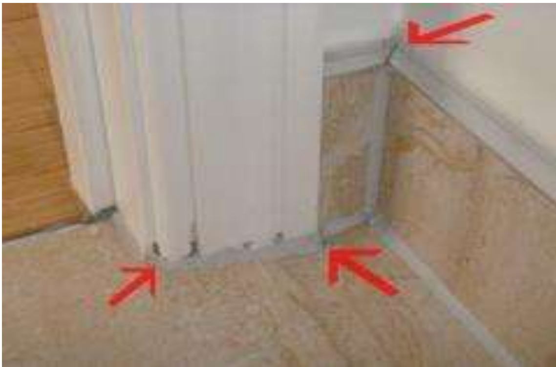
Poor finishing in toilet area.
