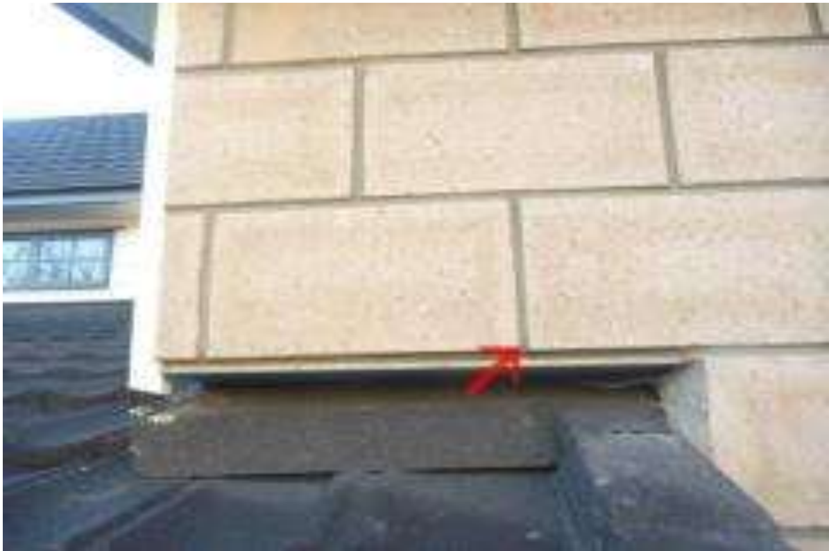
No weep holes in brick cladding on the lintel. Downpipe needs a spreader at the bottom.
