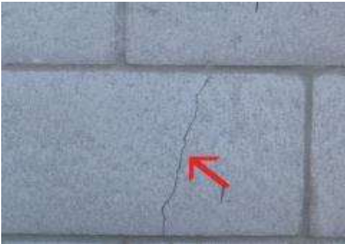
Cracked masonry block.
