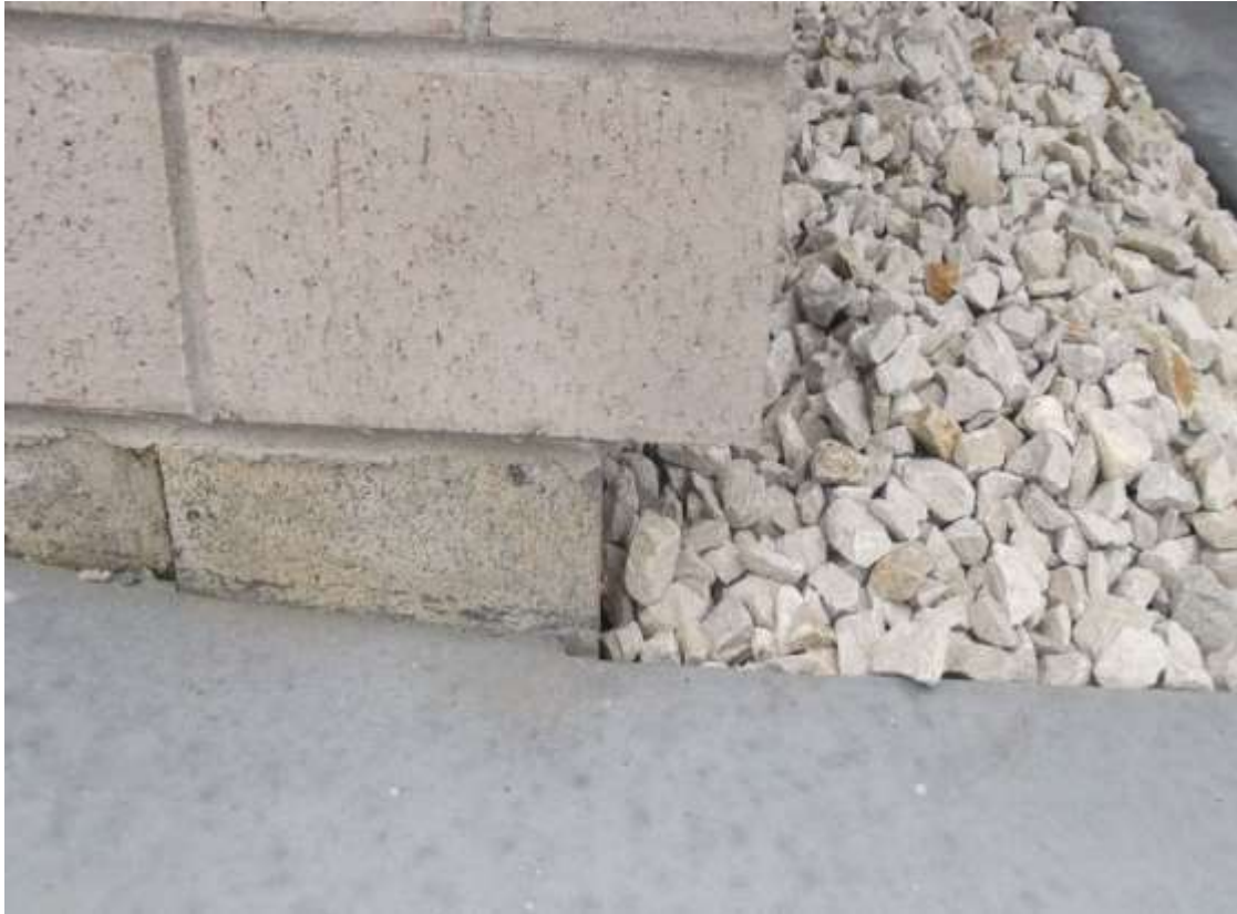
Poor foundation work, or alternatively blocks should have been cut to fit the slab.
