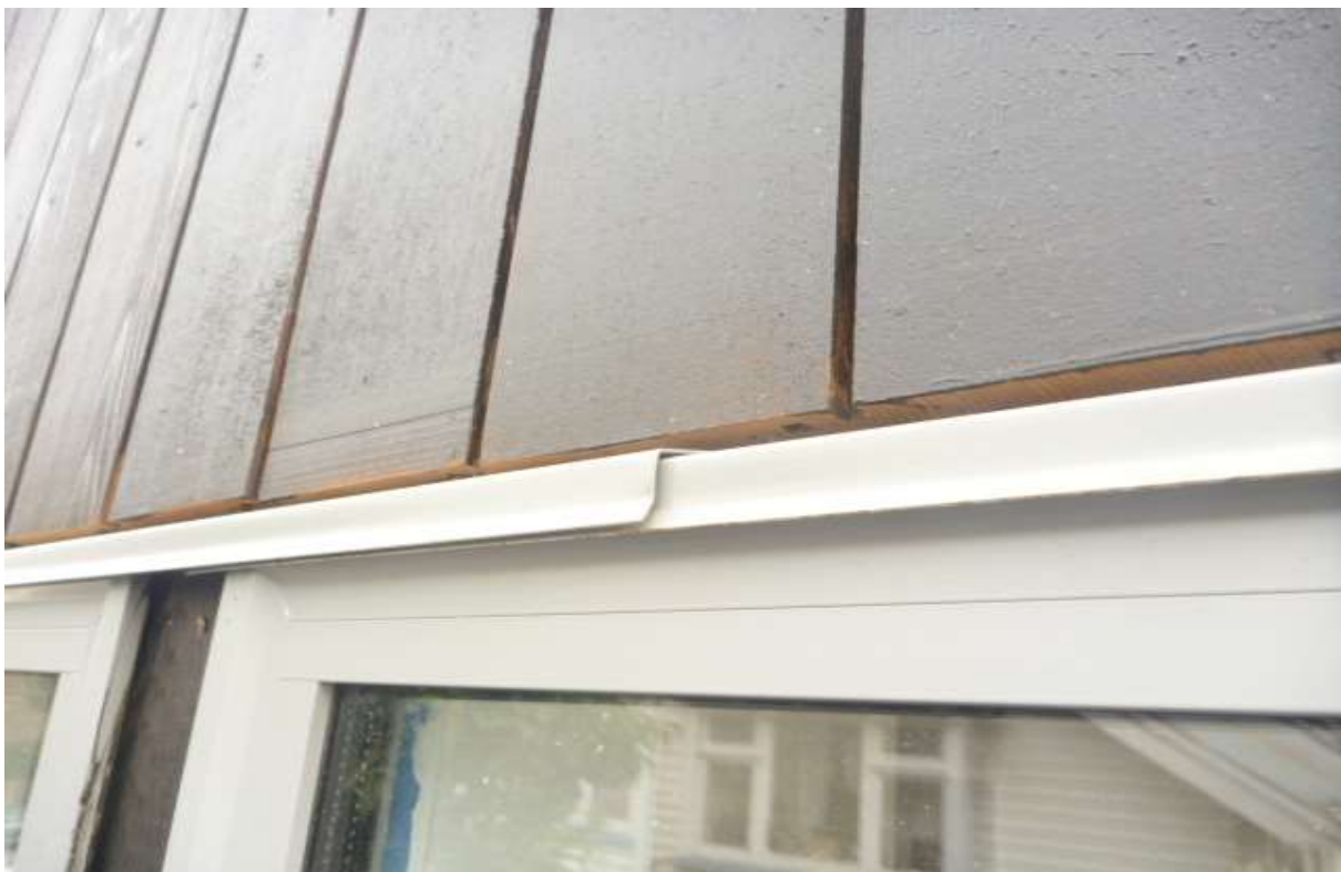
Poor junction of the flashing allowing moisture entry. Bottom edge of cladding needs painting.
