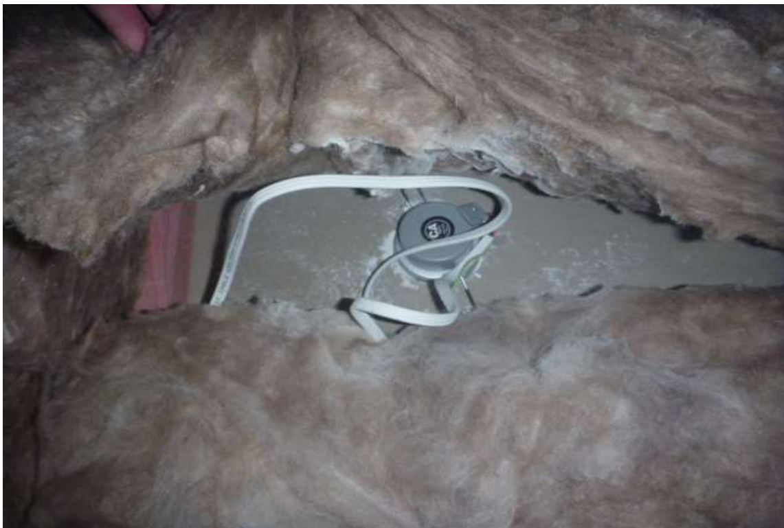
Excessive clearance. Downlight has a CA 135 mark so rated insulation could abut the can.
