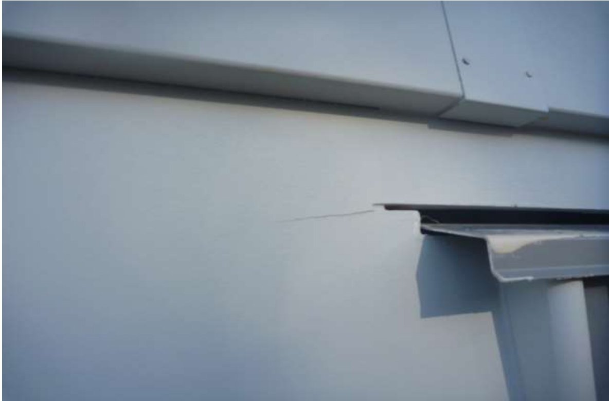
Over-cutting of weatherboard for the flashing. No stop-end was visible behind the cladding. Weatherboard is split.
