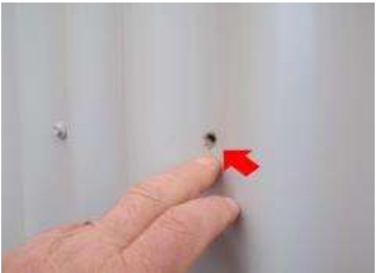
No sealing of hole on vertical corrugated sheet steel.
