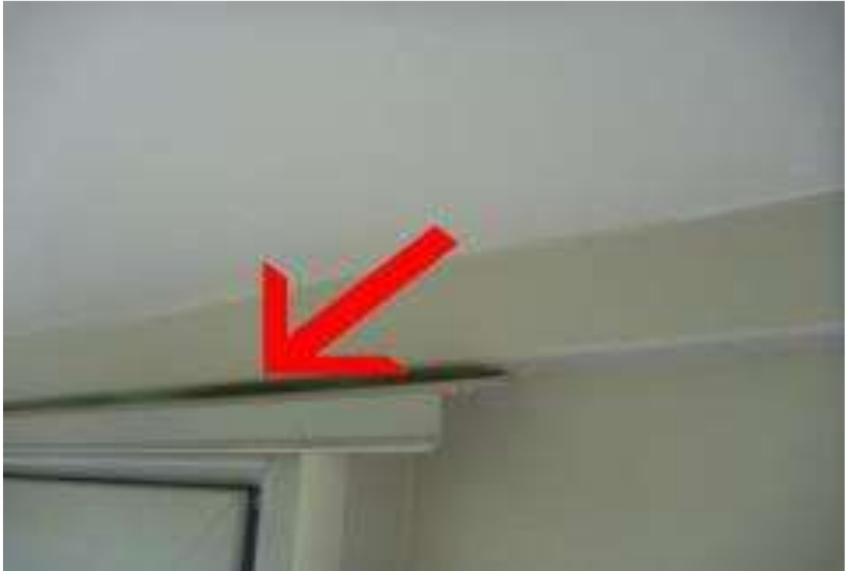
Inadequate clearance between cladding and head flashing
