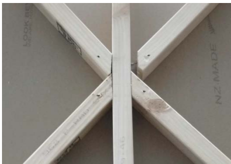
Figure 73. Centre joint in diagonal brace separating in Combo 1
