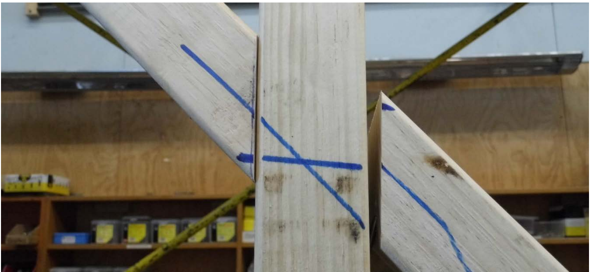
Figure 26. Brace in tension
