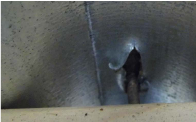
Figure 67. Views of sheet slotting at lead-head nails – vertical corrugated steel
