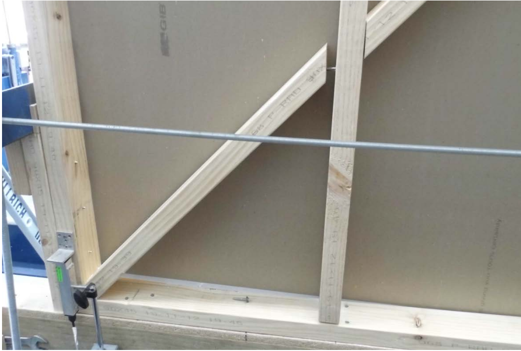
Figure 72. Diagonal braces separating in Combo 1
