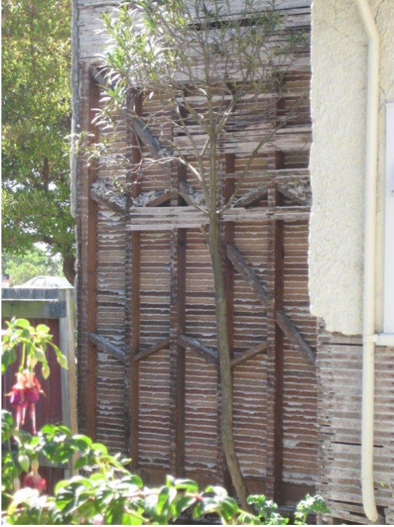
Figure 5. View of an earthquake-damaged lath and plaster exterior wall (Buchanan et al 2011)
