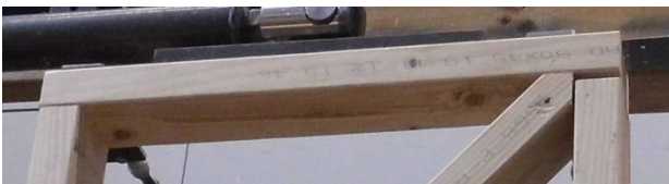
Figure 37. Top plate lifting in Brace 4 before strengthening
