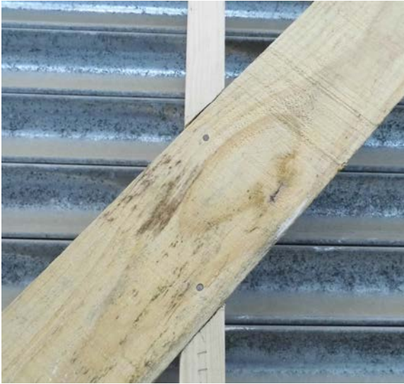
Figure 15. Joint at intermediate studs in specimen for 150 x 25 let in brace at 45°
