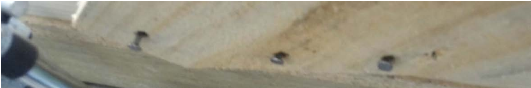
Figure 19. Nails pull out of diagonal brace connection
