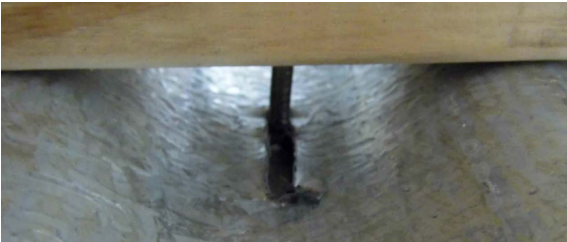
Figure 62. Views of sheet slotting at lead-head nails – horizontal corrugated steel
