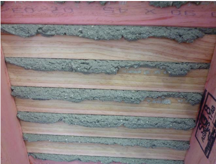
Figure 11. Plaster squeezed between laths
