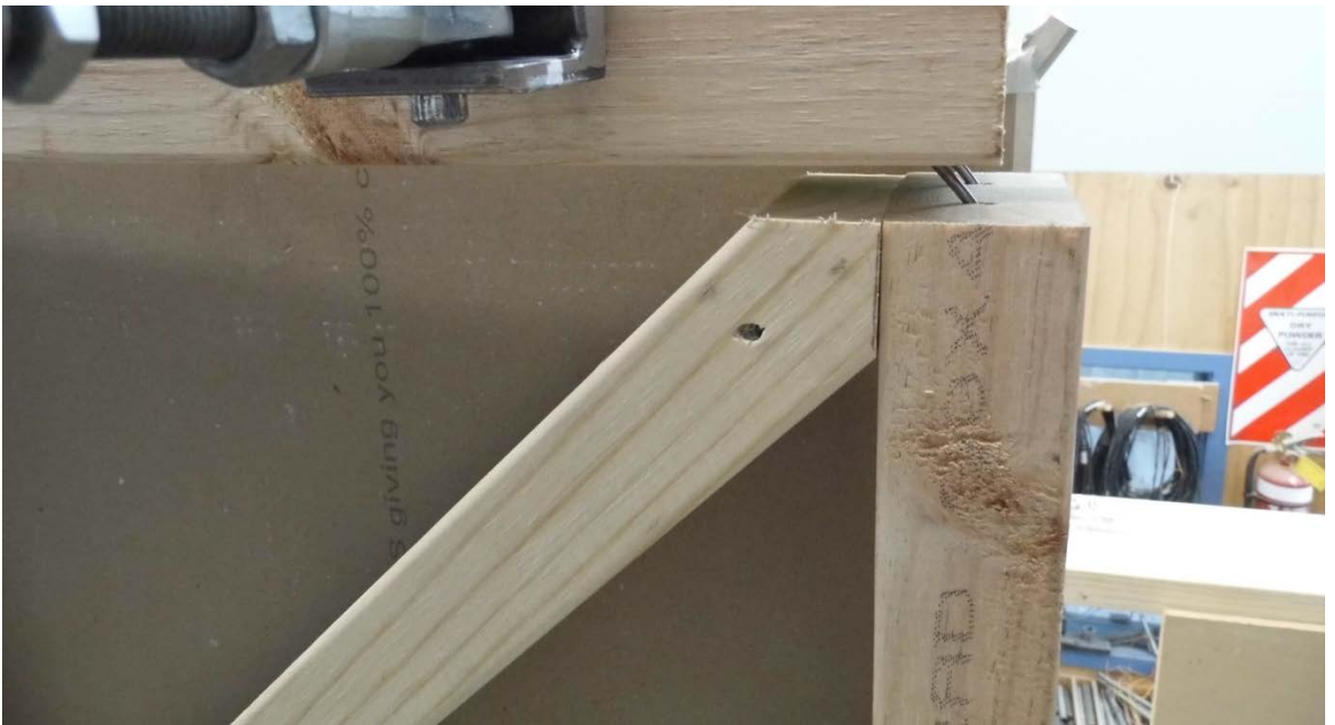
Figure 71. Top plate lifting in Combo 1
