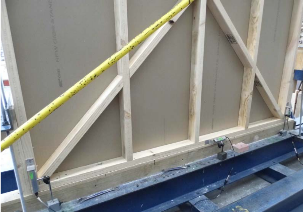
Figure 70. Double diagonal brace in Combo 1
