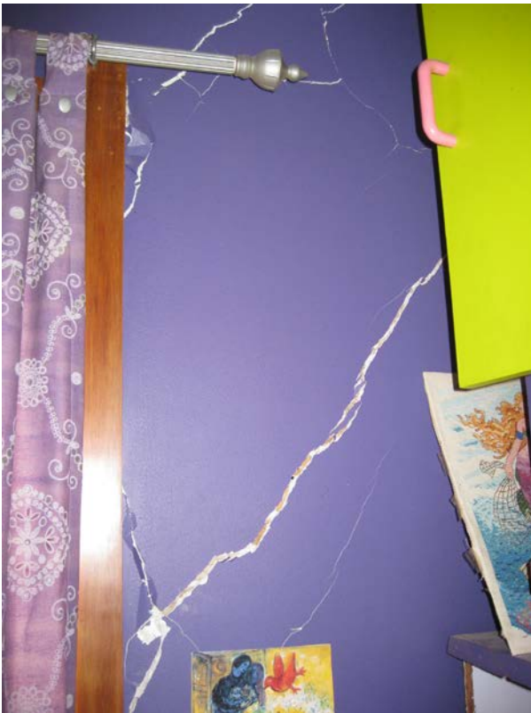
Figure 6. View of an earthquake-damaged interior lath and plaster wall (Buchanan et al 2011)
