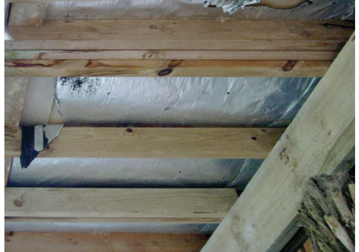
BRANZ has seen many cases where torn or damaged foil no longer provides effective insulation.
