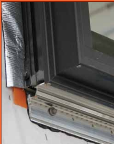
Support bar fixed to a sill trimmer under an aluminium window, cavity cladding.
