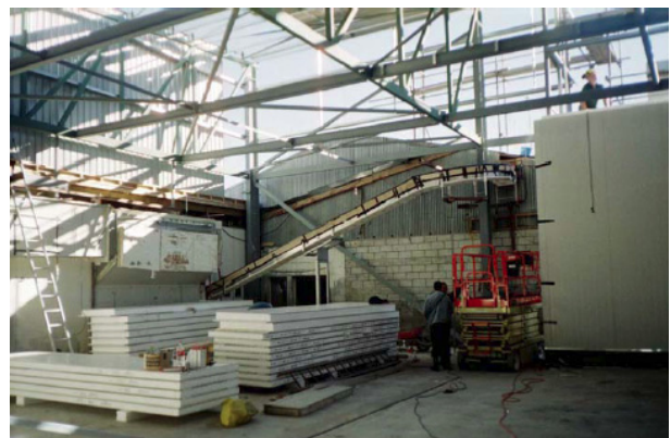
Specifying just enough product will help to make sure that it is not wasted on site.
