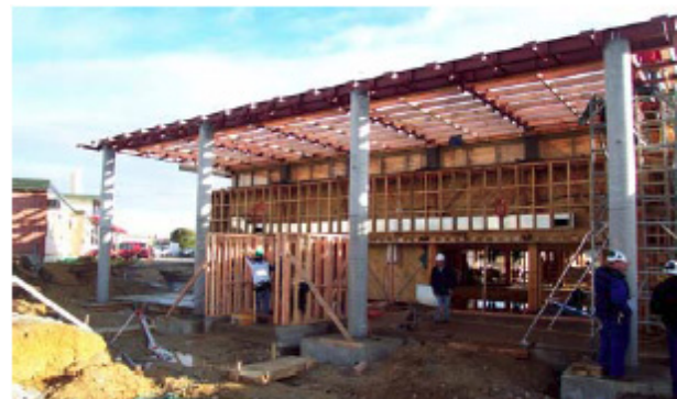
Use prefabricated framing to reduce timber off-cuts during the early stages of construction.
