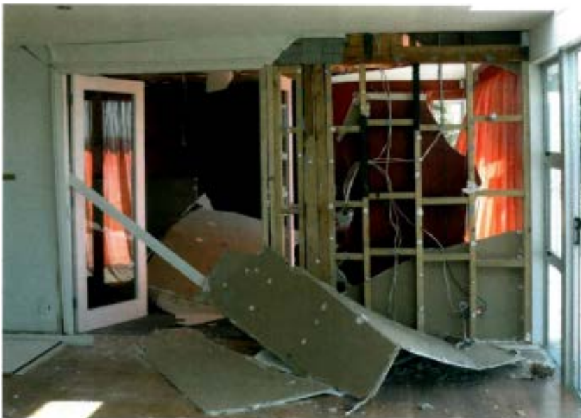
Figure 1 Severe failure of high-grade plasterboard internal linings (Buchanan et al. 2011)
