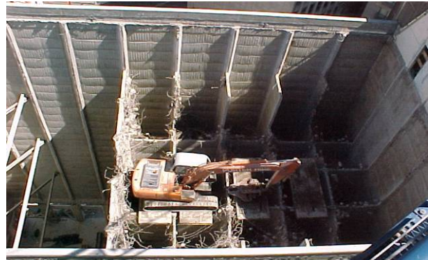
Dismantling the Northern Roller Mills building, Auckland floor by floor (Ward Demolition).
