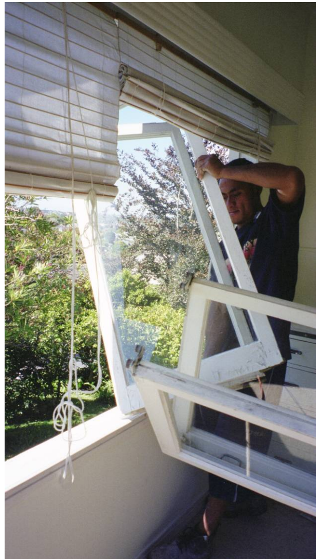
Dismantle good-quality building parts carefully for reuse on your project or for resale (Ward Demolition).
