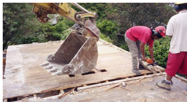
Ward Demolition removing wooden floor boards from a house and salvaging the timber.
