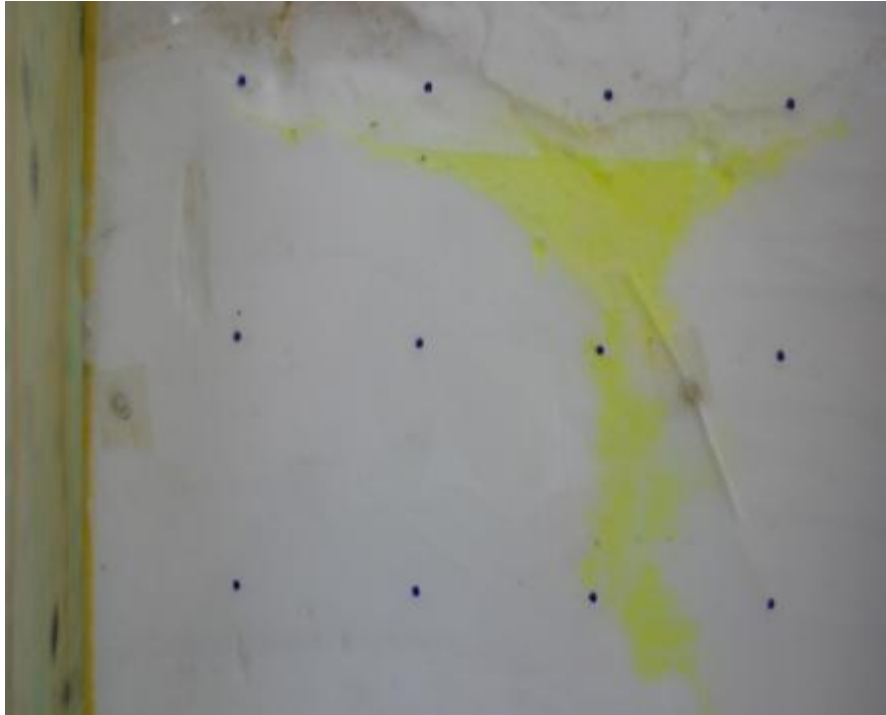
Figure 4: Leakage well established 43 minutes after start of test (D4864)
