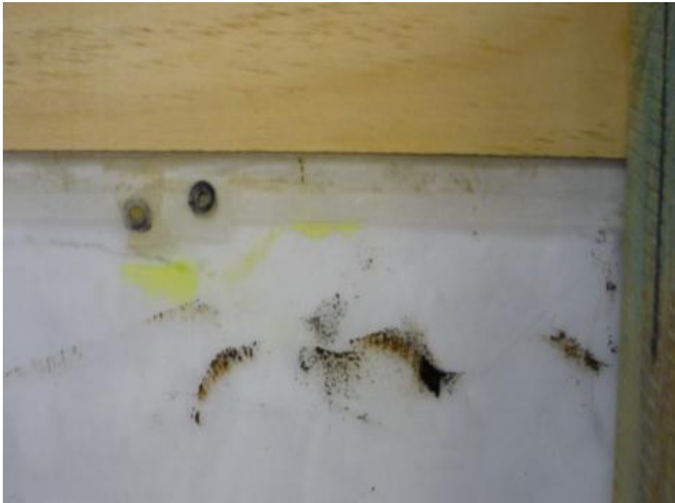
Figure 2: Leakage observed 2 minutes after start of test (D4864)
