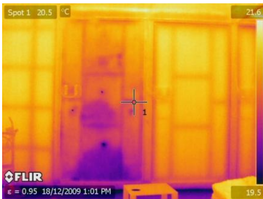
Figure 6: Thermal image of brick veneer test sample during drying stage after Airfoam installation
