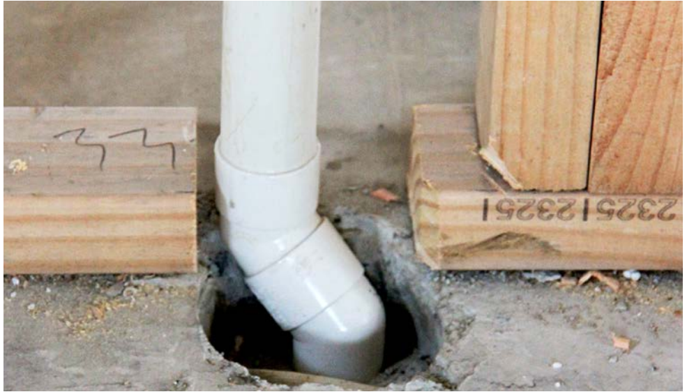
Cutting out the bottom plate to fit services is not acceptable.
