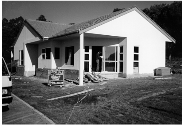
FIGURE 3. Front View of Whiby House during construction (note datalogger hut lower right).
