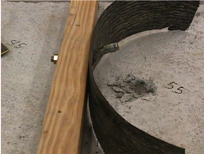
Photograph 5. Failure mode D
