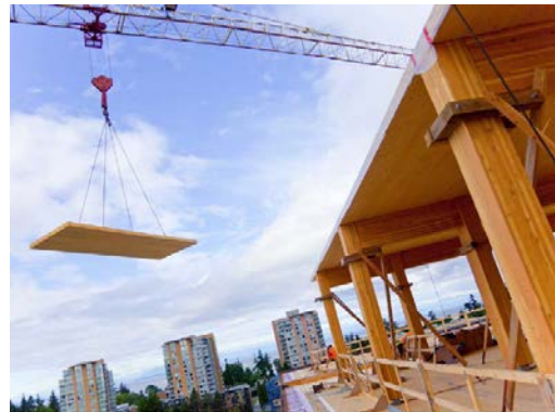
Figure 23: CLT timber can be used for walls, floors, roofs and structural members (Proefrock, 2011).
