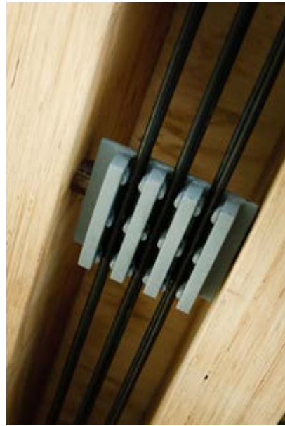
Figure 19: The post-tensioned LVL beams in the CoCA building at Massey University, Wellington, are the first of their kind in the world (Massey University of Wellington, 2012).
