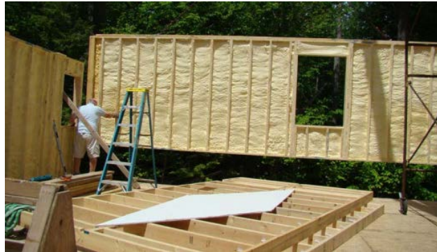
Figure 20: An open panel wall being put into place onsite (Davis Frame Co., 2012).
