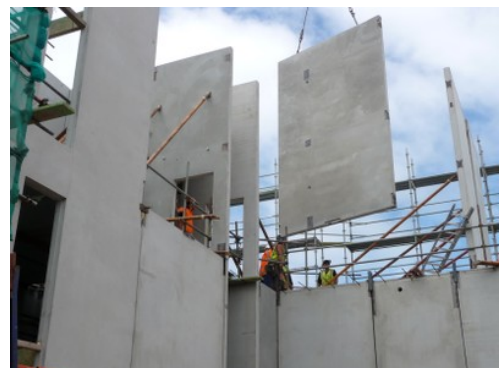
Figure 25: Precast concrete panels are craned into position and fixed in place (Charleson, 2012).
