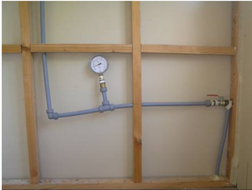
Figure 5: Inlet to house with pressure gauge.
