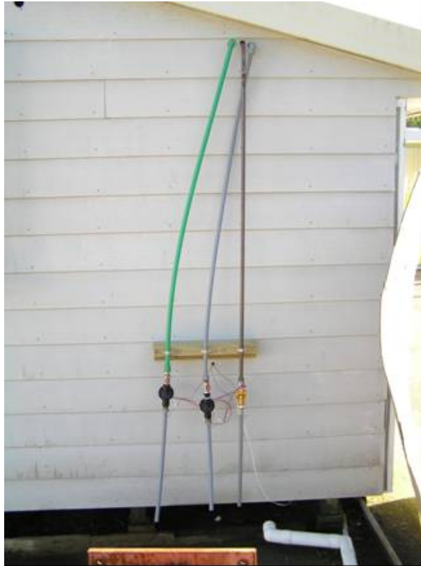
Figure 6: Outlet of the three distribution pipes with solenoid valves.
