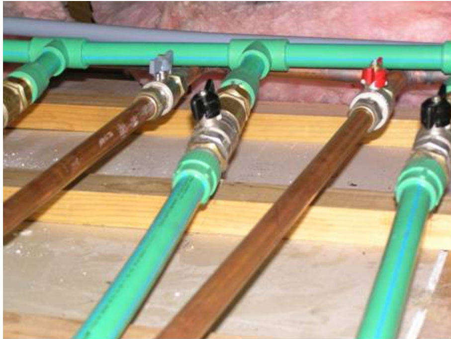
Figure 8: Range pipe connection to main distribution pipes for PP-R (green) and Cu (brown) range pipes. PB (gray) distribution pipe in background.
