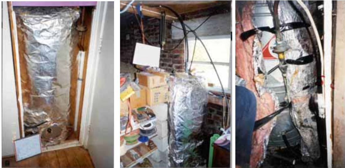
Figure 168: Examples of electric hot water cylinder wraps
