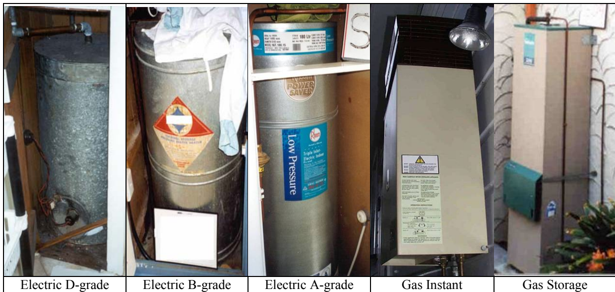
Figure 55: Examples of hot water cylinders
