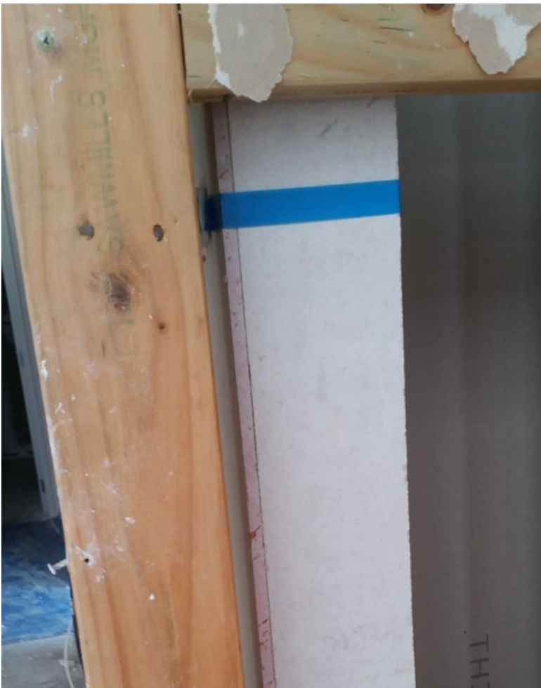
Figure 60. Plasterboard bulkhead held together with combustible plastic strapping.
