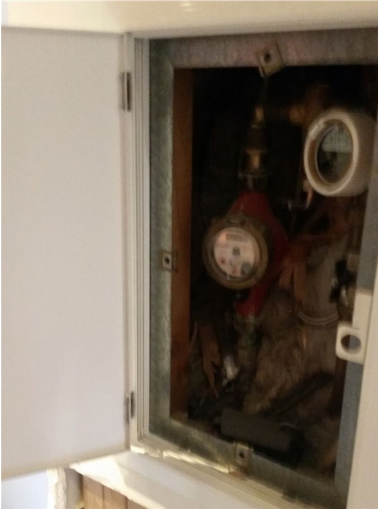
Figure 64. Non-rated access hatch into a full-height service shaft.
