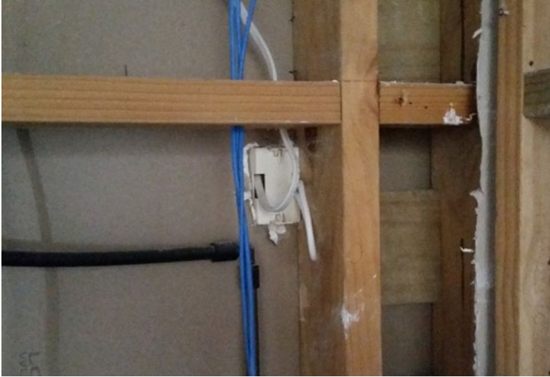
Figure 61. Unrated flush boxes in fire-rated walls.
