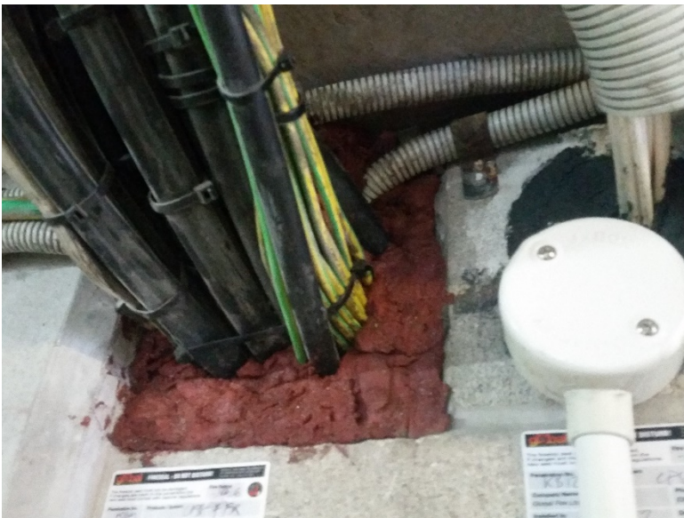
Figure 65. Multiple large cable bundles without stopping between bundles.
