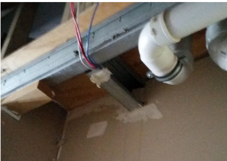
Figure 63. Non-sealed structural steel penetration of a fire-rated wall.
