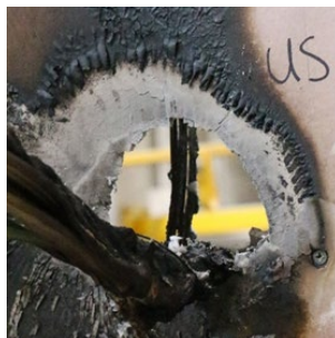
(c) Unexposed post-test
