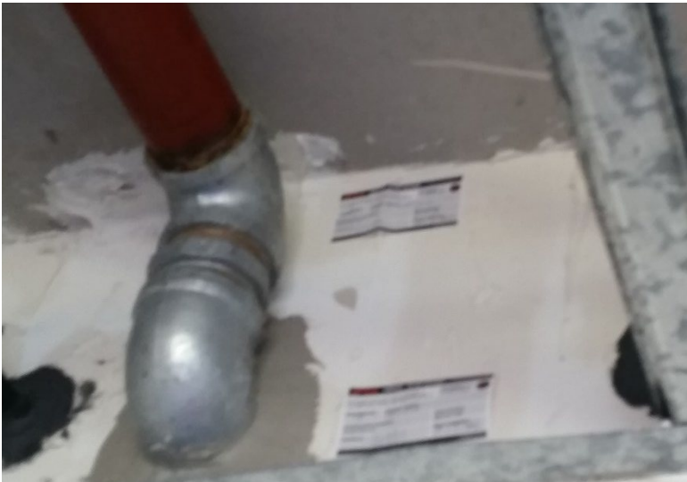
Figure 62. Penetrations through fire walls sealed with smoke seal only.
