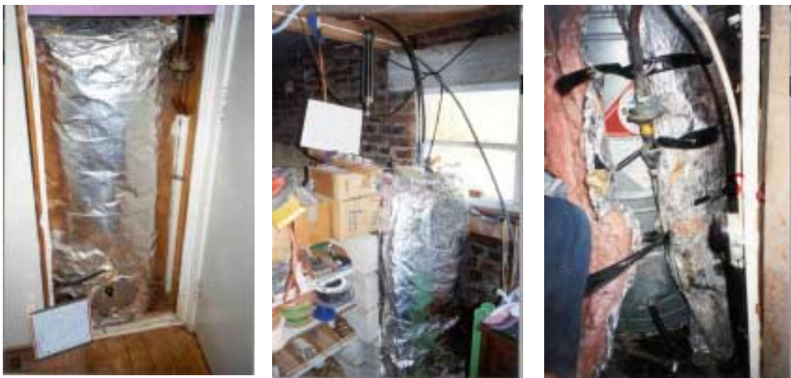
Figure 17: Examples of electric hot water cylinder wraps
